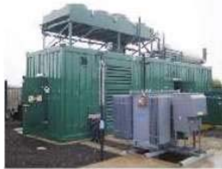
Fig. 2.4. Internal combustion generator fueled by methane gas.
