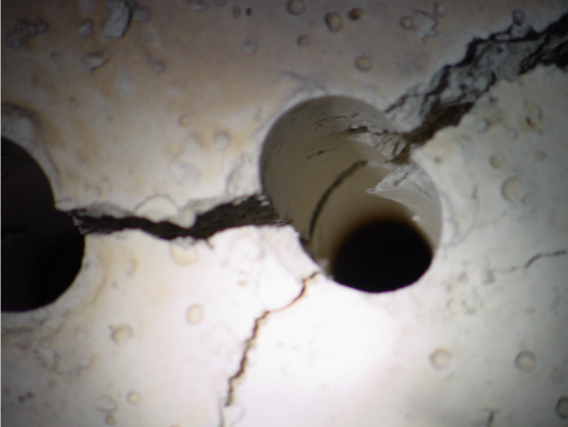
Figure 47 Enlargement showing critical delamination failure at 5-6" in depth and accompanying transverse cracking.
