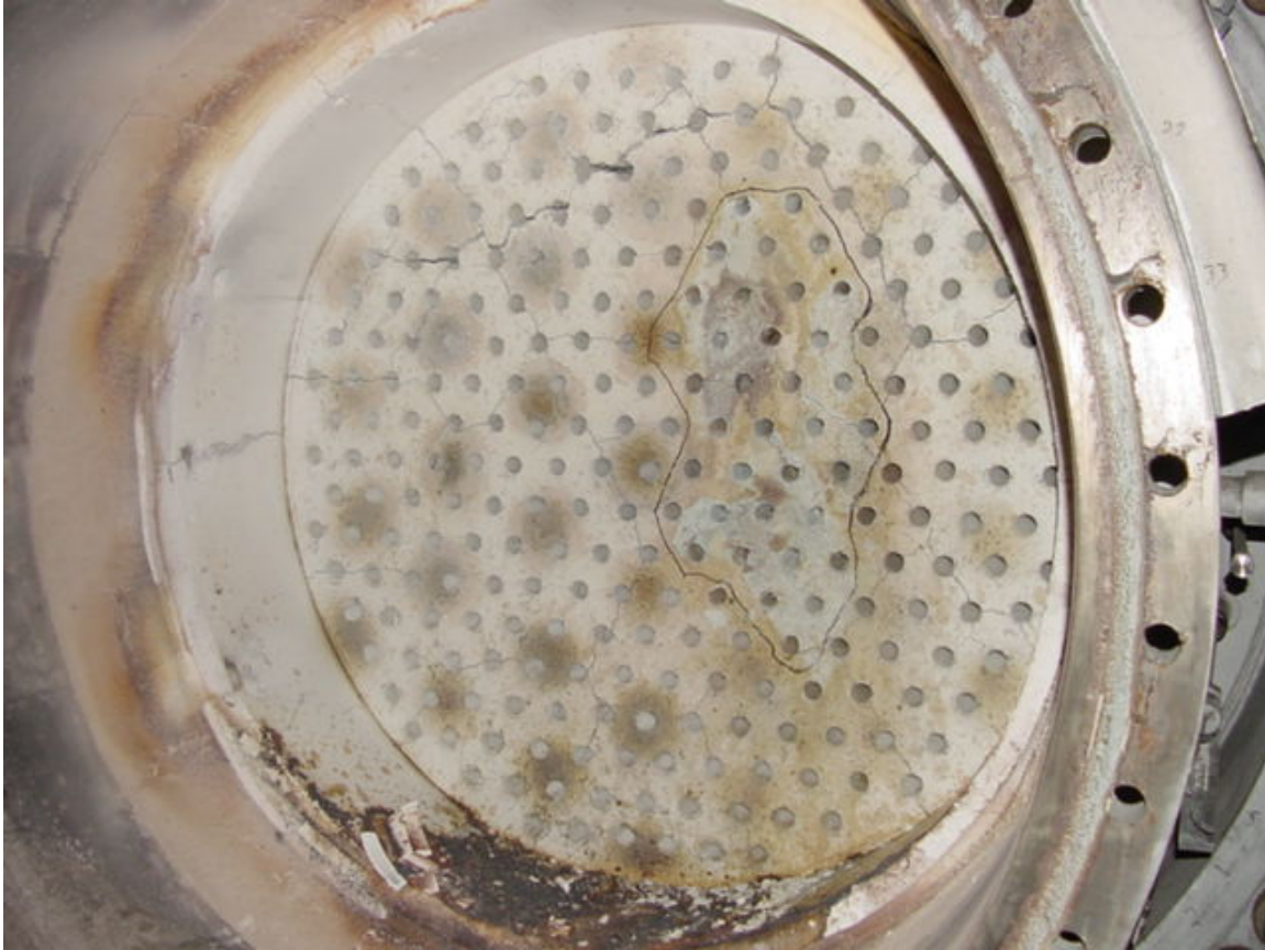
Figure 46 Picture of failed pulse combustor tube sheet.
