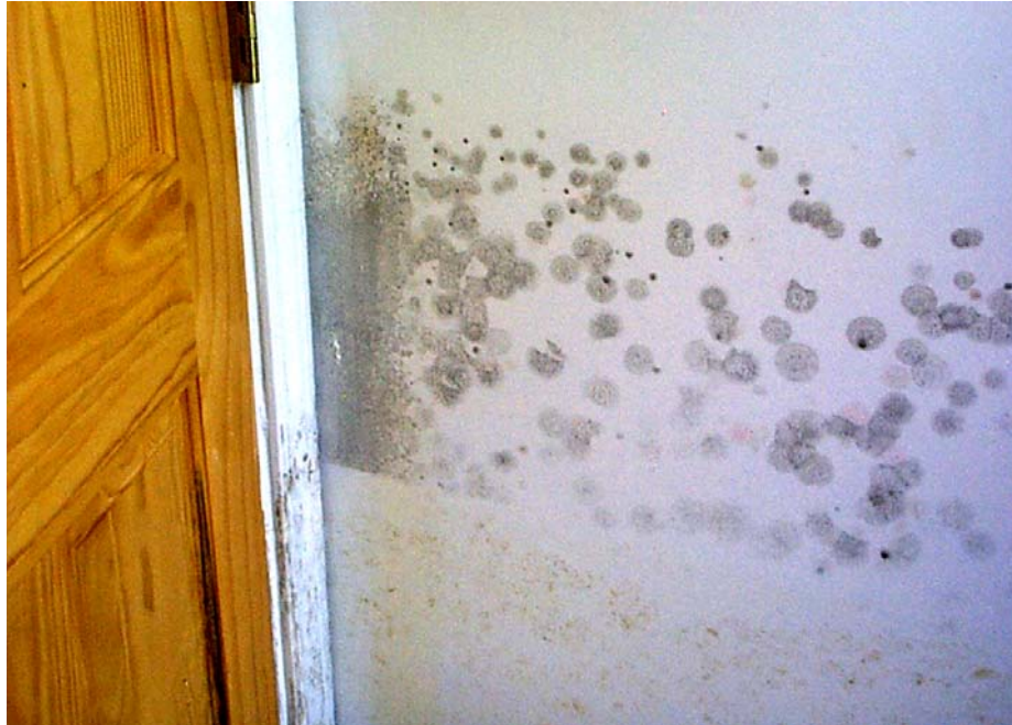
Figure 5-6 Module S-2 (Wall 4) Day 10 - After washing with water. Mold growth and staining on walls
