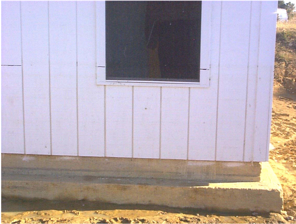
Figure 4-15 Module S-1 (Wall 1, North Exterior Wall) Post-flood, Day 8 (before washing). Walls are stained below flood level.
