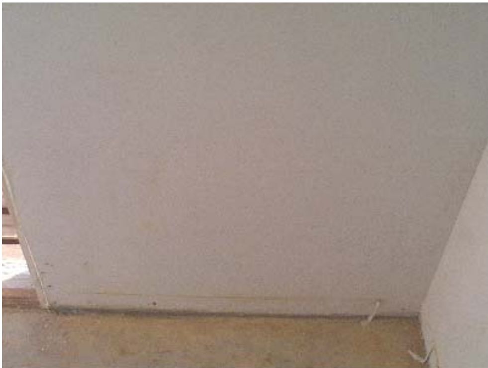
Figure 6-10 Module S-3 (Wall 3) Day 15 - After sanitizing. No mold visible
