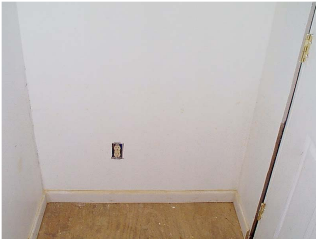
Figure 6-14 Module C-3 (Wall 2) Day 15. No sanitization occurred and no mold growth appeared; wall is restorable.
