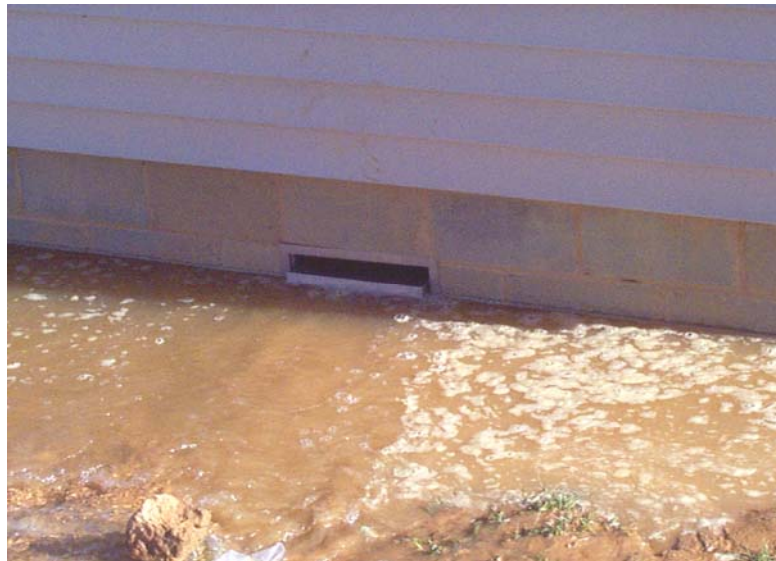
Figure 6-5 Module C-3. Water draining out of open crawlspace flood vents
