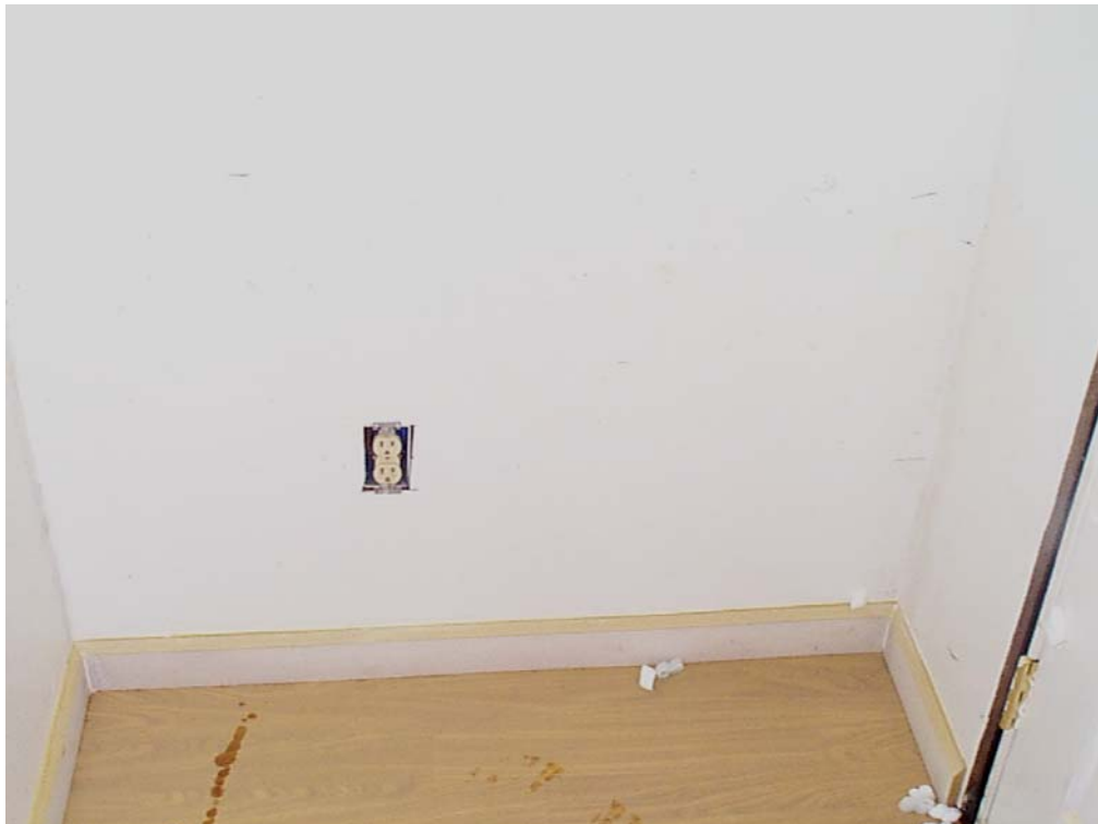
Figure 6-12 Module C-3 (Wall 2) Day 8 – Before washing. Note: “Pellets” on the floor at right bottom are Styrofoam which was placed on the floor of the unit prior to flooding. As floodwater rose, the pellets floated, and cameras could record locations where water appeared to flow into the unit.
