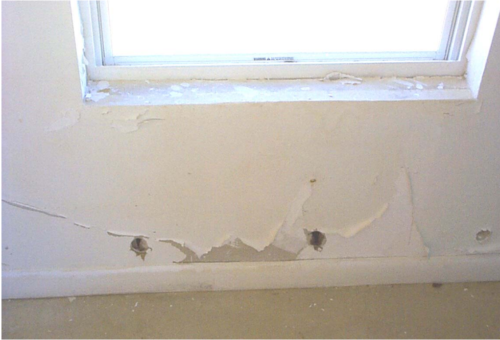
Figure 4-7 Module S-1 (Wall 1) Post-flood, Day 29. Little change in wall staining and paint peeling has occurred.
