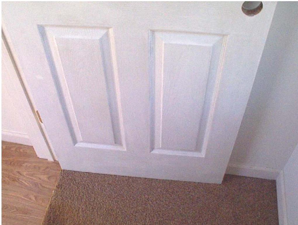
Figure 6-15 Module C-3 Interior door – Pre-flood. Door is in new condition.
