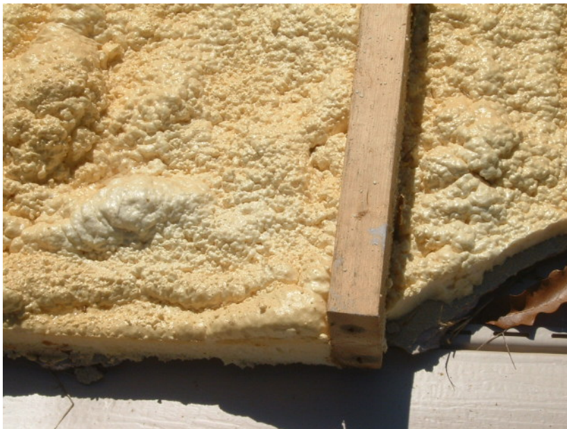
Figure 6-40 Module C-3, Wall 3, Interior. No mold or severe staining was observed at autopsy which occurred 15 months after the flood test.
