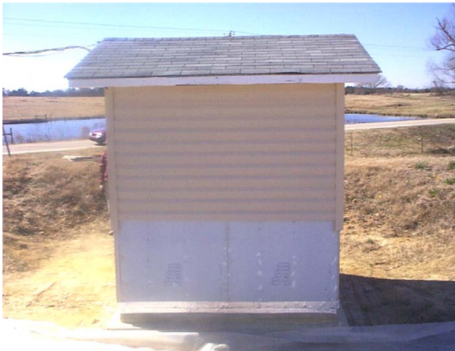
Figure 6-32 Module S-3a, east wall with adhesive sealant tape installed. Prior to flooding
