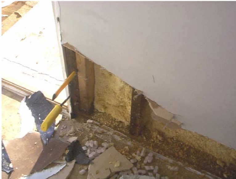
Figure 6-36 Module S-3a Interior south wall after second dry flood proof test. Water entered the module during flooding through the crack between the doubled studs (yellow knife and saw) that form the door rough framing.
