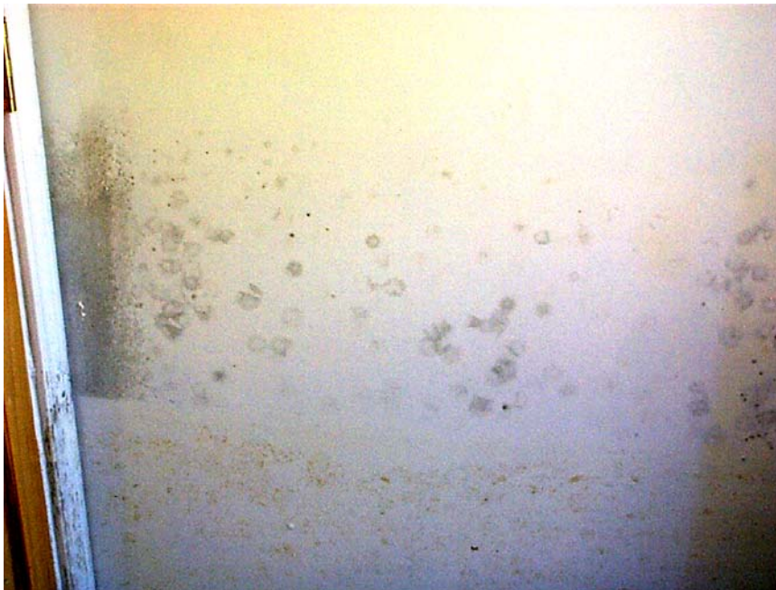
Figure 5-5 Module S-2 (Wall 4) Day 8. Mold growth and staining on walls
