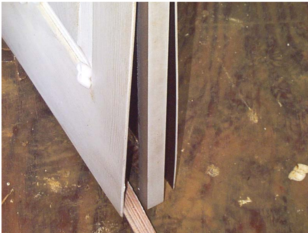
Figure 6-16 Module C-3 Interior door – Day 8. Door surface is delaminating.
