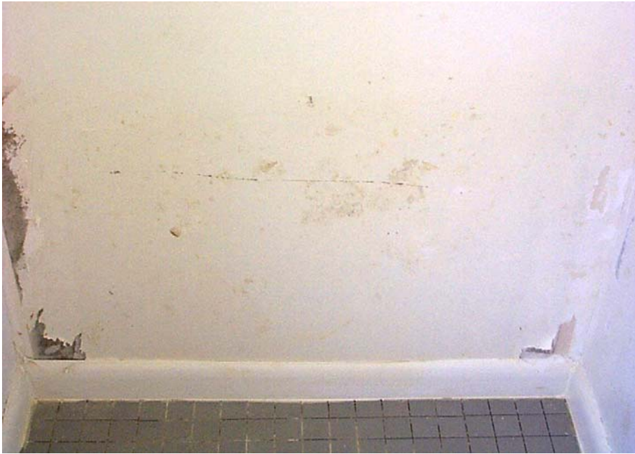
Figure 5-12 Module C-2 (Wall 2) Day 15 after sanitizing. Staining remains, mold growth disappears
