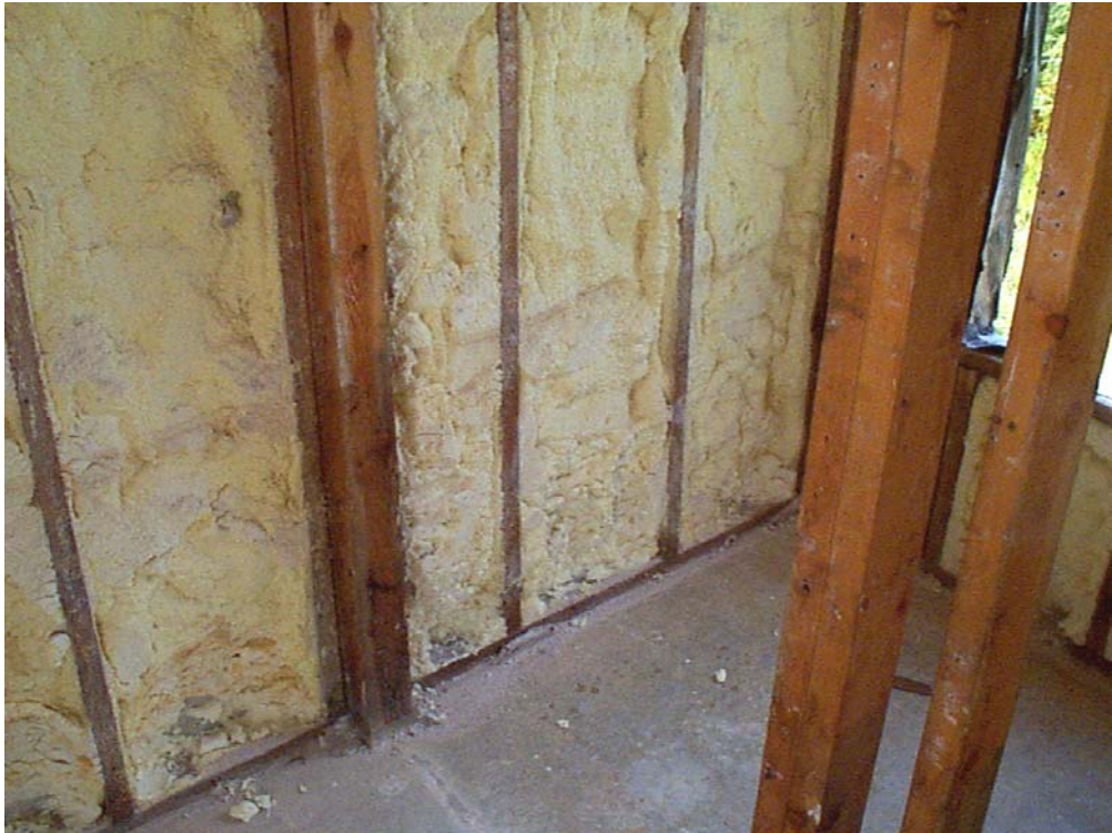
Figure 6-17 Inside of Module S-2 (Wall 4) at autopsy. Insulation and wall cavities are dry and in good condition
