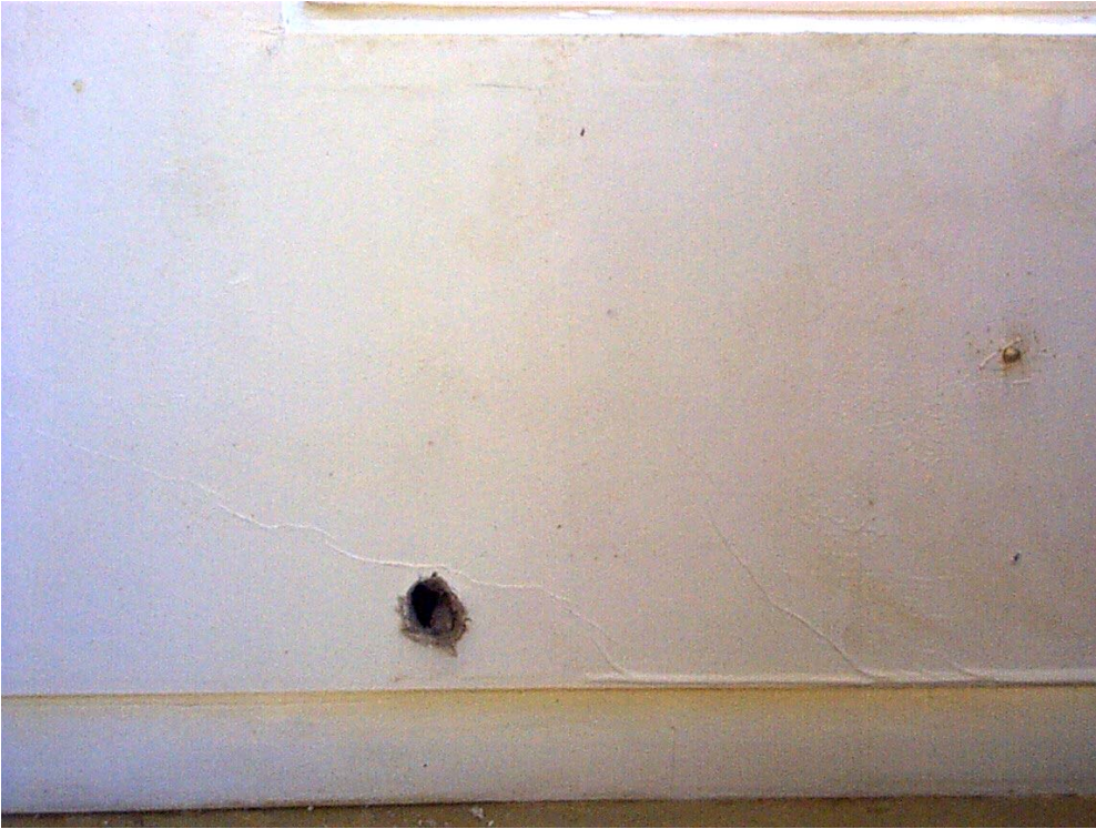
Figure 4-5 Module S-1 (Wall 1) Post-flood, Day 8 - Before washing. Hole punched in lower wall to aid cavity draining; walls are stained; paint is sagging and rippling.
