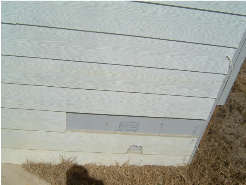
Figure 6-39 Module C-3, Wall 2, Exterior. No mold or severe staining was observed at autopsy which occurred 15 months after the flood test.
