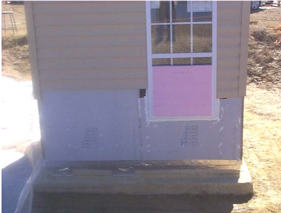
Figure 6-31 Module S-3a, north wall with window dam and adhesive sealant tape installed. Prior to flooding
