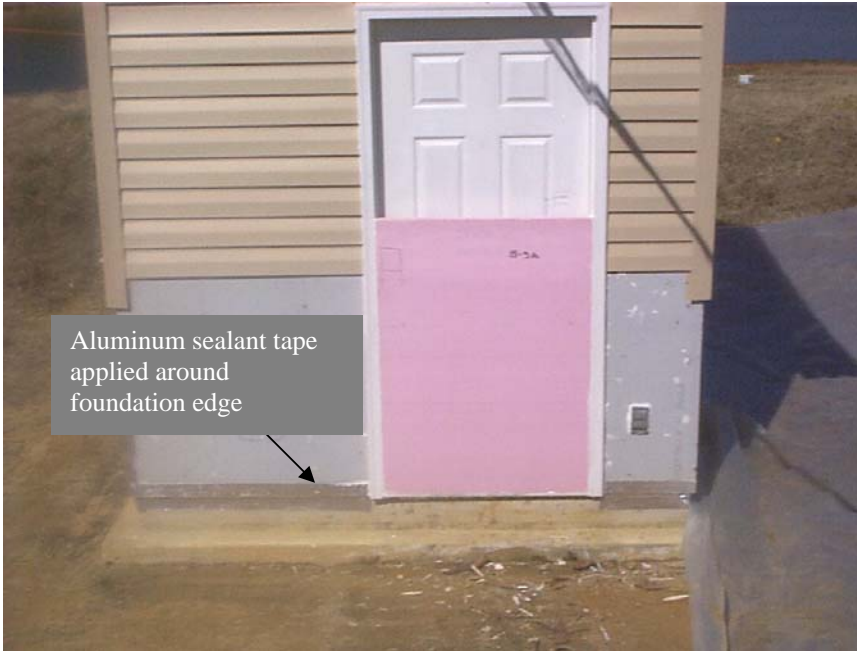
Figure 6-29 Module S-3a, south wall with door dam and aluminum/butyl rubber adhesive sealant tape installed. Prior to flooding
