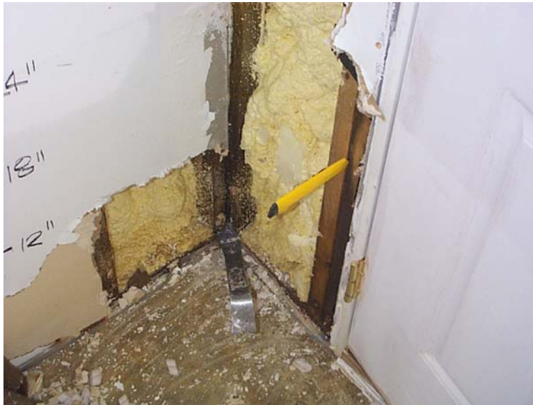
Figure 6-35 Module S-3a Interior southeast corner of Room S-301 after second dry flood proof test. Water entered the module during flooding through the crack between the doubled studs (yellow knife) that form the door rough framing. It also entered through the crack between the corner studs and the sill plate (grey pry bar).
