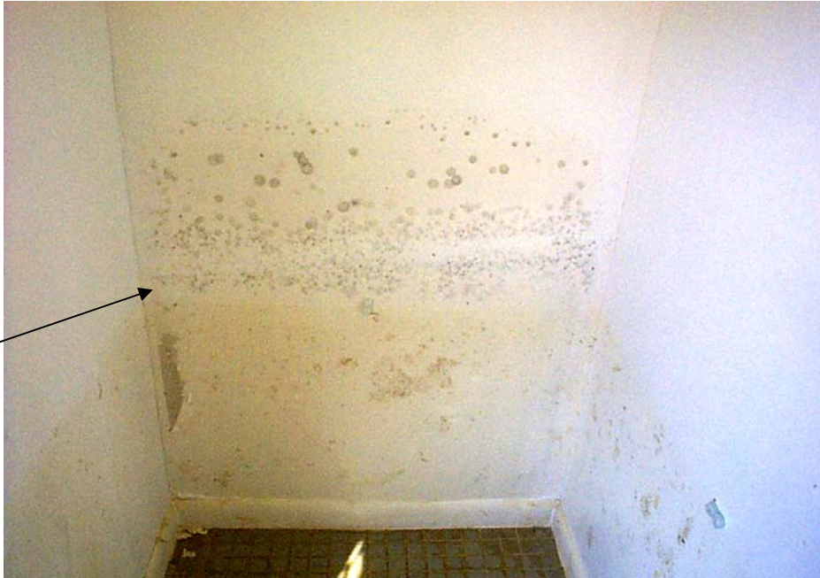
Figure 5-10 Module C-2 (Wall 2) Day 8 at re-entry. Wall is stained and mold growth observed
