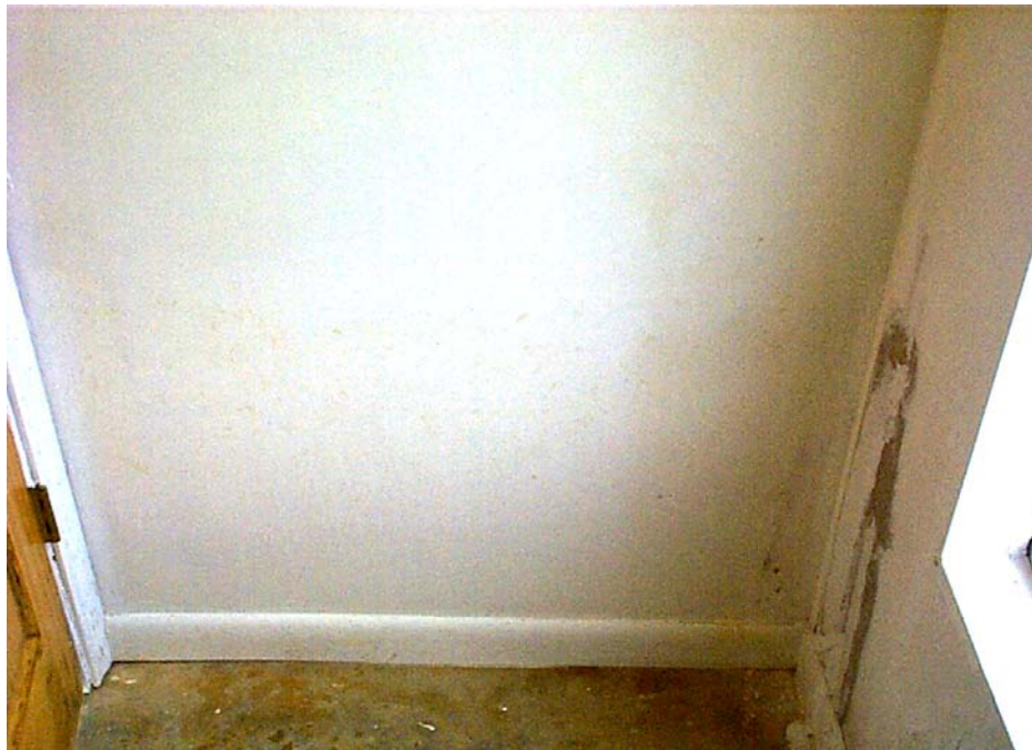
Figure 5-7 Module S-2 (Wall 4) Day 15 - After sanitizing. Mold discoloration gone, some staining remains
