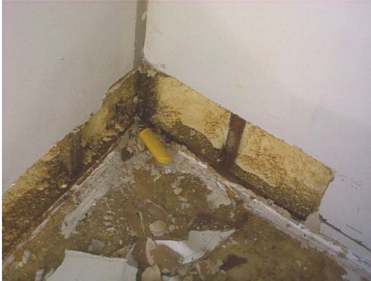
Figure 6-37 Module S-3a Interior southwest corner of Room S-301 after second dry flood proof test. Water entered the module during flooding through the crack between the corner studs and the sill plate (yellow saw).
