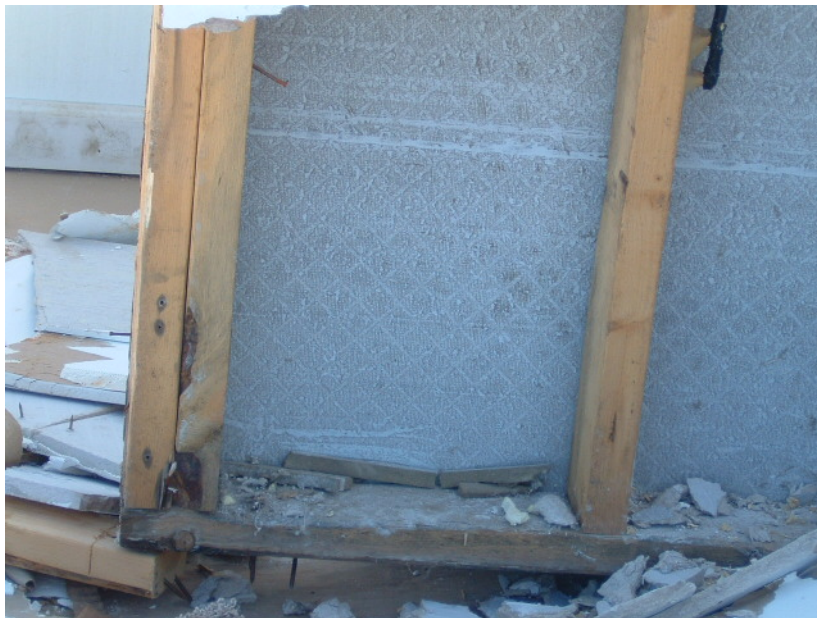
Figure 6-42 Module C-3, Wall 5, Interior. No mold or severe staining was observed at autopsy which occurred 15 months after the flood test.
