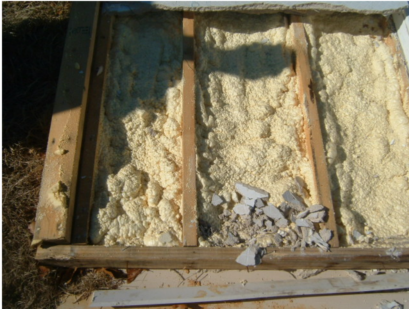
Figure 6-41 Module C-3, Wall 4, Interior. No mold or severe staining was observed at autopsy. The grey debris in the lower portion of the photo is the remains of the interior wall board.
