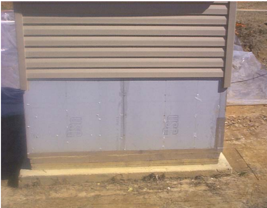
Figure 6-30 Module S-3a, west wall with adhesive sealant tape installed. Prior to flooding
