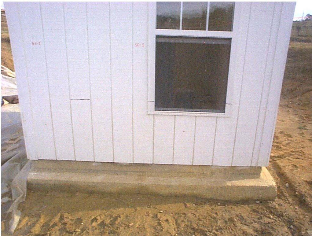
Figure 4-16 Module S-1 (Wall 1, North Exterior Wall) Post-flood, Day 15 (after washing). Wall remains slightly stained.
