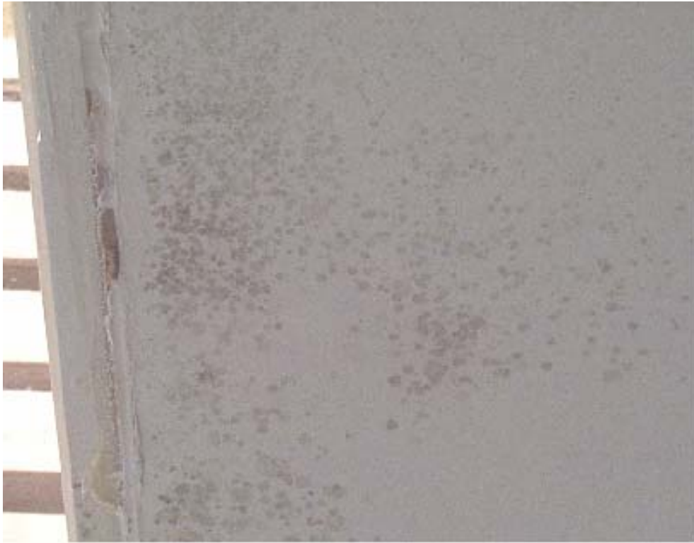
Figure 6-9 Module S-3 (Wall 3) Day 10 - After washing with water. Mold remains
