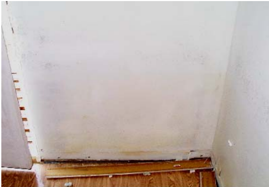
Figure 6-8 Module S-3 (Wall 3) Day 8 – Before washing. Wall is stained and there is mold growth.
