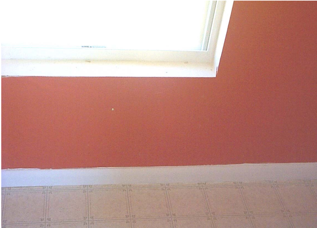
Figure 4-9 Module C-1 (Wall 1) Pre-flood. Vinyl wall covering, vinyl floor cover, and window are in new condition.
