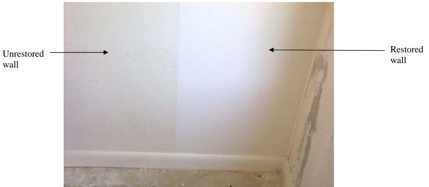
Figure 5-8 Module S-2 (Wall 4) After Restoration. Wall is restorable. Although the fiber reinforced gypsum interior panels shown here on Wall 4 of Module S-2 supported mold growth due to flooding, sanitization and restoration efforts have brought the general appearance back to almost its original state.
