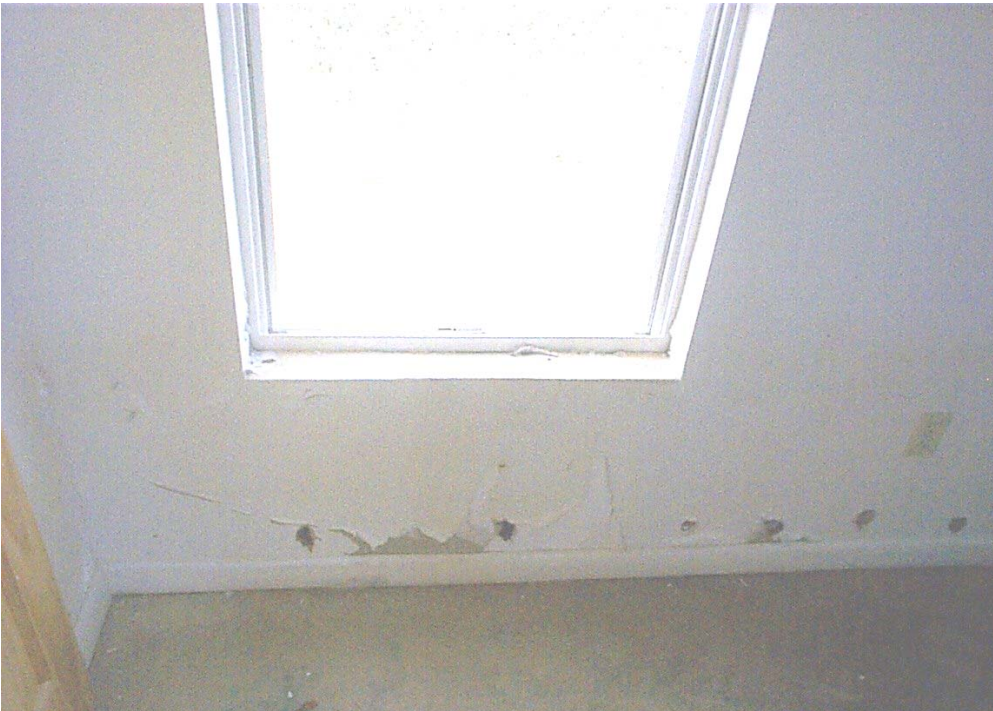
Figure 4-6 Module S-1 (Wall 1) Post-flood, Day 15. Walls stained and paint peeling; no mold growth
