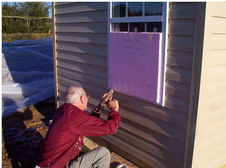
Figure 6-1 Module S-3 Placement of flood proofing dam over window. Two beads of adhesive sealant were applied to seal the Styrofoam dam and then additional caulking was placed around all the sides.
