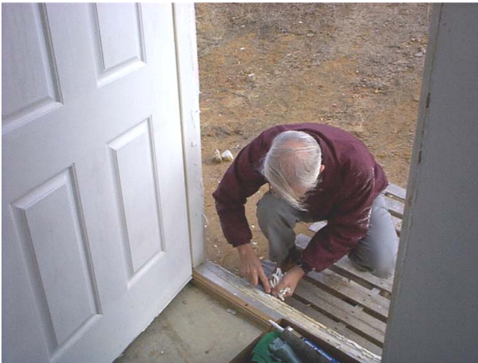
Figure 6-28 Silicon II caulking was installed on the threshold. Prior to reinstalling the polystyrene foam flood dams
