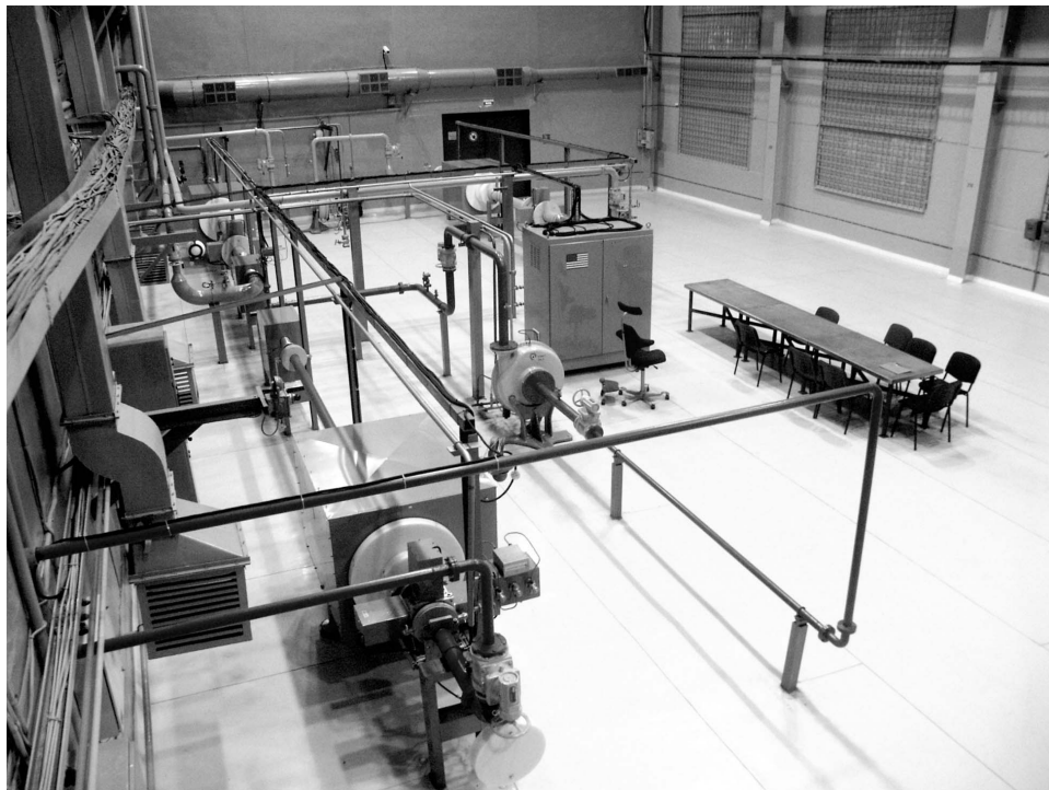
Fig. 26. BDMS equipment in the SChE Enrichment Plant BDMS room (installed in October 2004). Source: V. Afanasyev et al., "Installation of the Blend Down Monitoring System at the Siberian Group Of Chemical Enterprises, Seversk, Russia," 46 th Annual Meeting of the INMM , Phoenix, Arizona, July 20, 2005.
