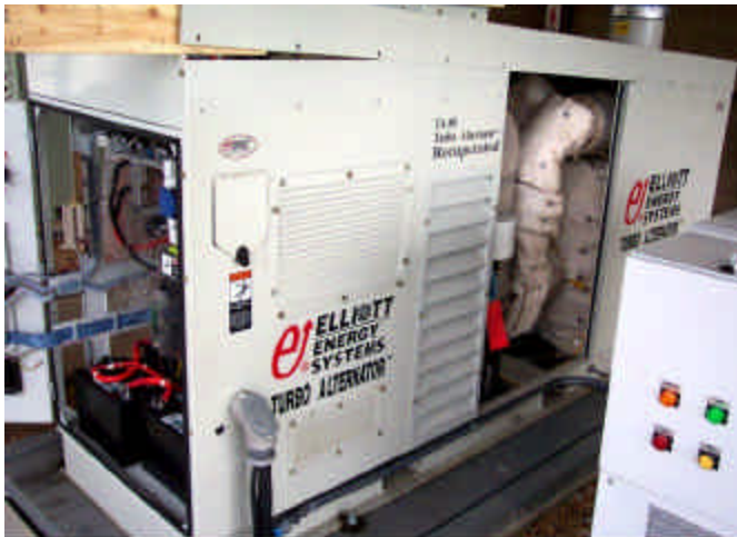
Elliott microturbine (80kW) opened for servicing
