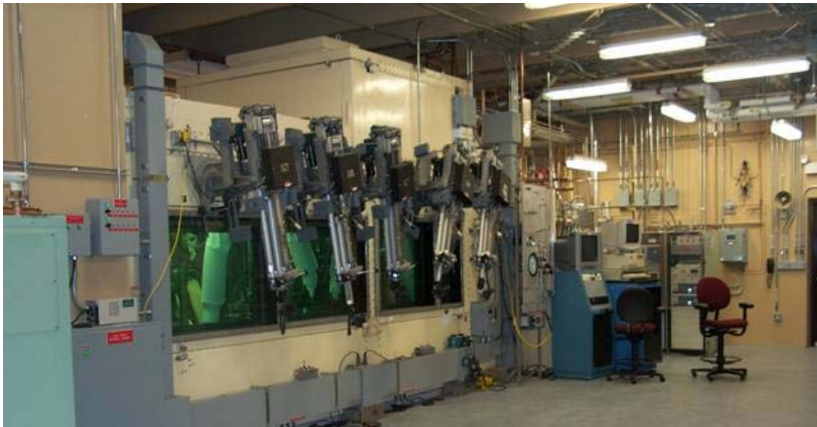
Figure 6. IAAC assembly/loading glovebox.
