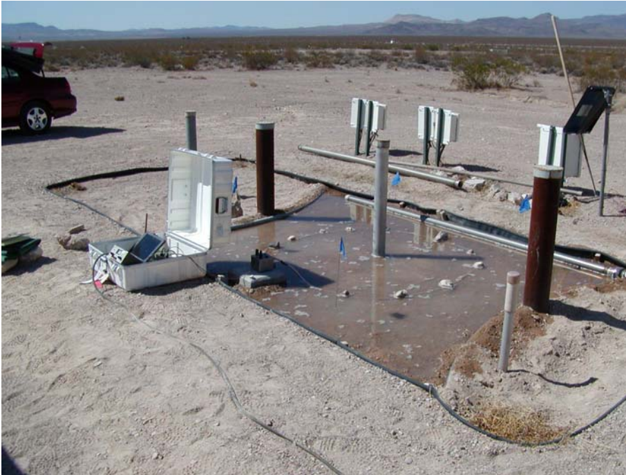
Figure 3. INL wireless sensor platform field test. For this test, the buried sensor packages (marked by the blue flags) are located on the exterior of the antenna encircling the aluminum well casing.
