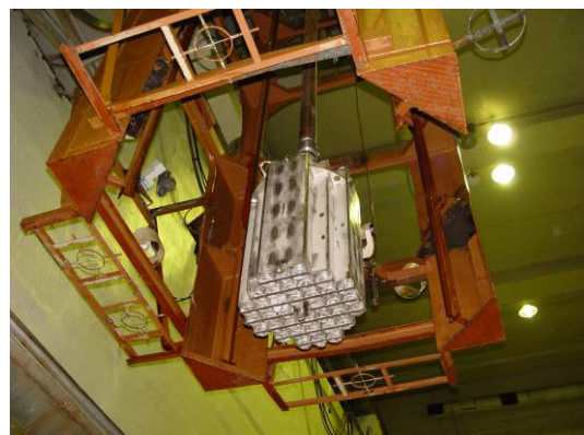
Figure 10. Loaded VPVR/M cask basket being transferred into the Building 101A hot shop/pool area.
