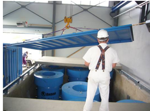
Figure 8. High-Level Waste Storage Facility extension cask storage vault.
