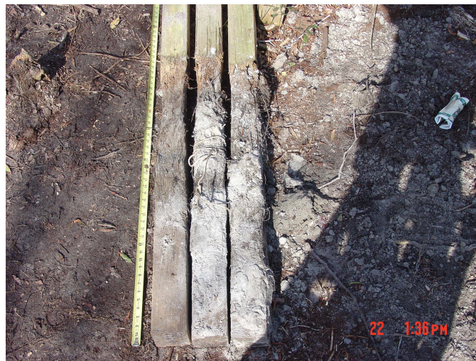
FIGURE 4 - Excavated posts showing deterioration
