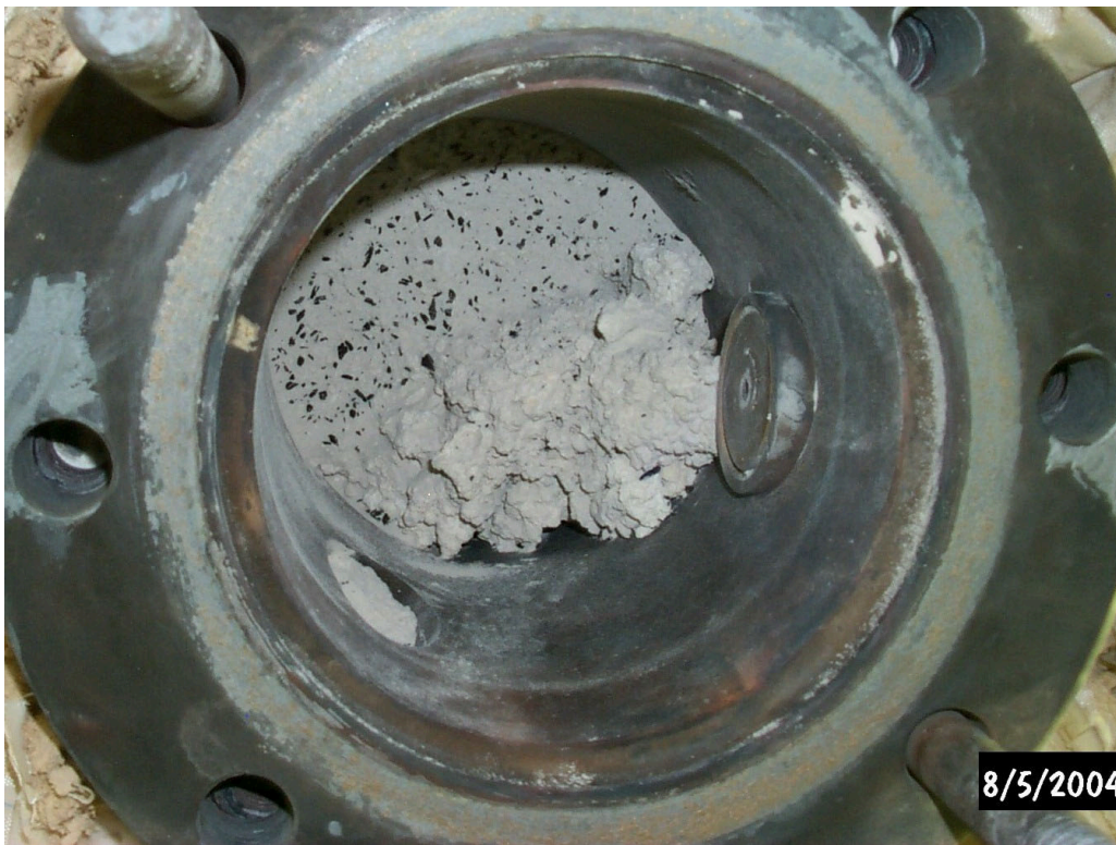
Figure 4.1-3. Bridged solids above the feed port, looking up through the bottom of the fluidized bed vessel.
