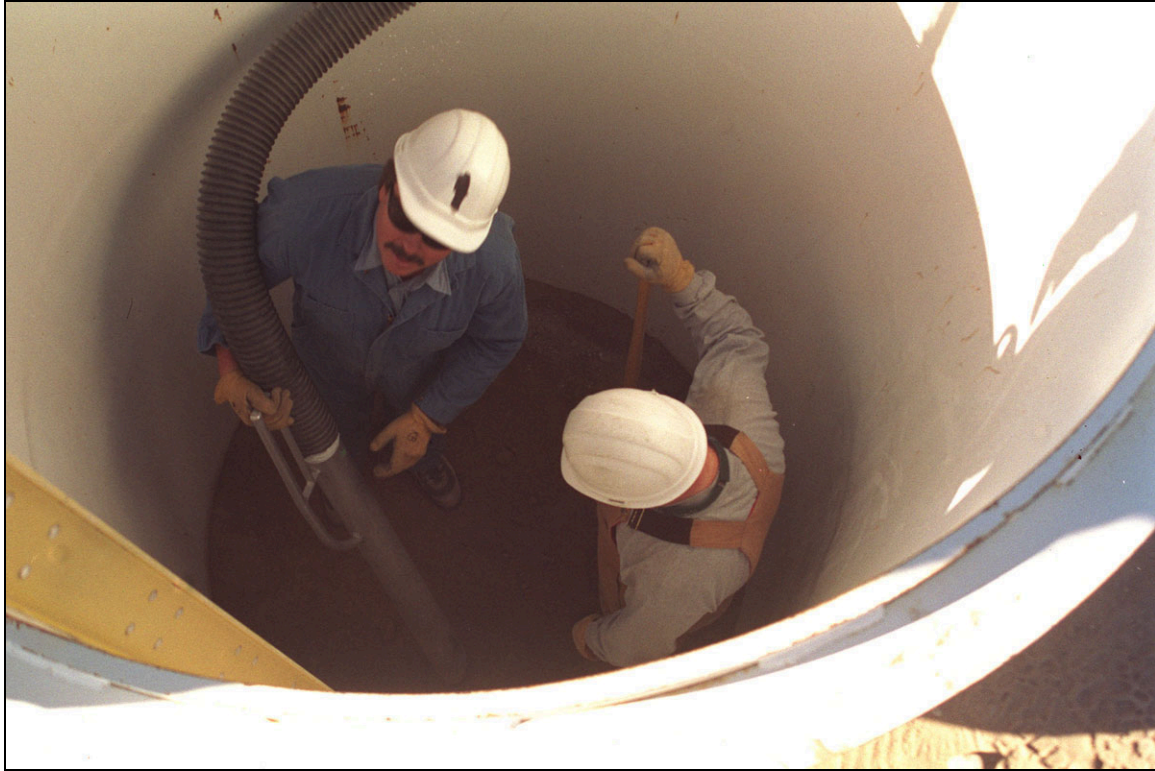
Figure 2-7. Soil Vacuum extraction – hose end. Workers vacuum soil while in the cave-in-protection sleeve.
