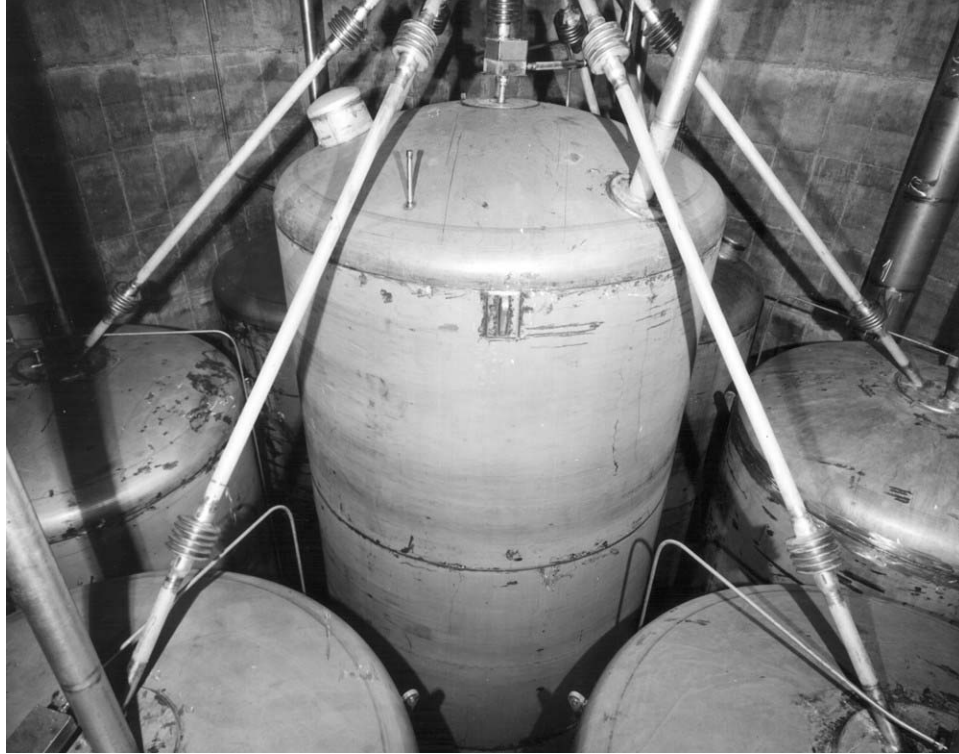
Figure A-4. Center Bin VES-WCS-139 (also known as VES-WCS-140-7) in interior of Calcined Solids Storage Facility III (71-4954).
