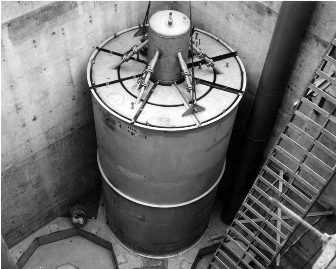
Figure A-2. Calcine storage Bin VES-WCS-115-2 in Calcined Solids Storage Facility I (59-5283).
