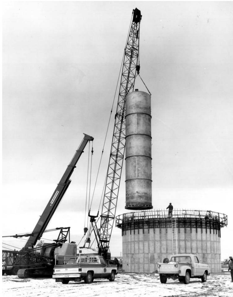
Figure A-5. Installation of Bin VES-WS4-142 in Calcined Solids Storage Facility IV (76-4518).
