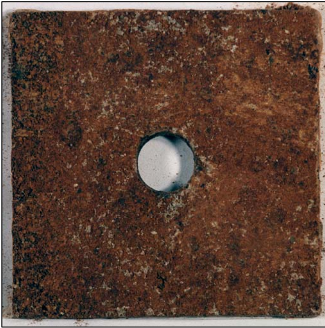
FIGURE 3 - Carbon Steel Coupon Before Cleaning, 6-year exposure at 3.05-m
