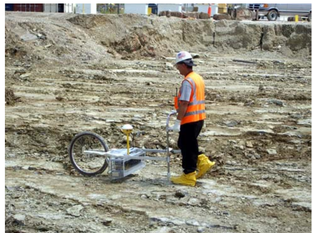
Figure 5. INL AXISS system deployed at the MCP Building-38 excavation site in Miamisburg, Ohio.
