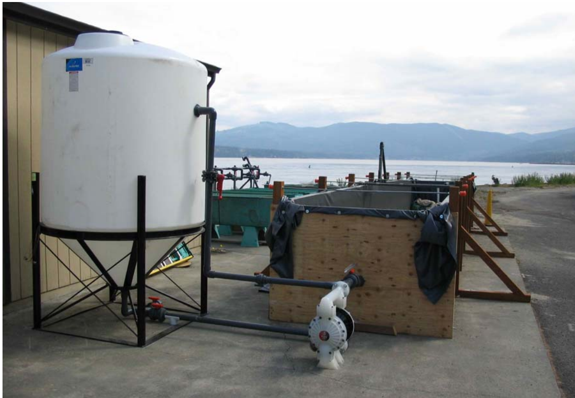
Figure 3. Slurry mixing tank, original pump, and surge current flume
