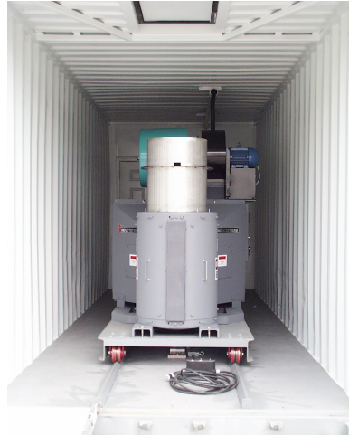
DEH Furnace on Cart
