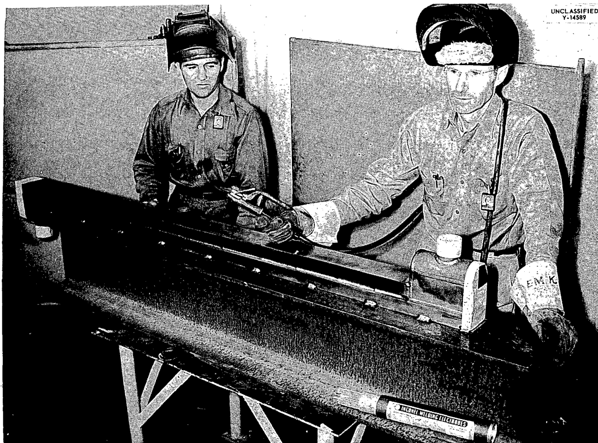
Fig. 43. Tube Bundle of Intermediate Heat Exchanger No. 2 After Completion of Root-Pass Weld on Pressure Shell. Note heavy strongback used to minimize distortion. (Secret with caption)
