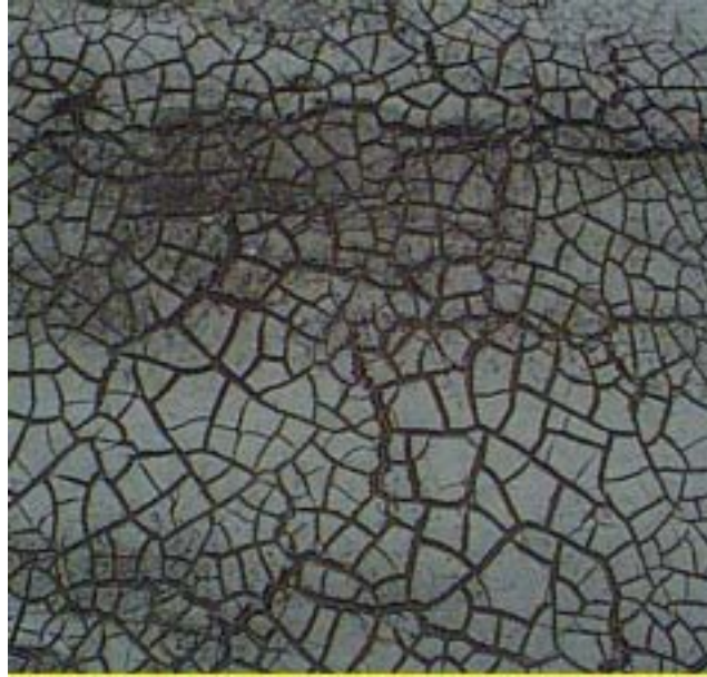
Cracks extend through one or more plies. High Severity
