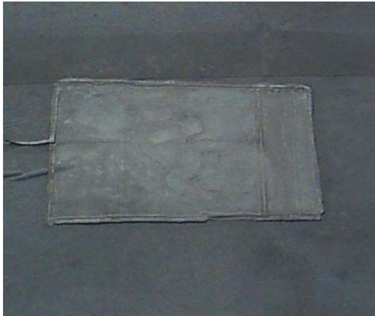
Temporary membrane patching different type of material. Medium Severity
