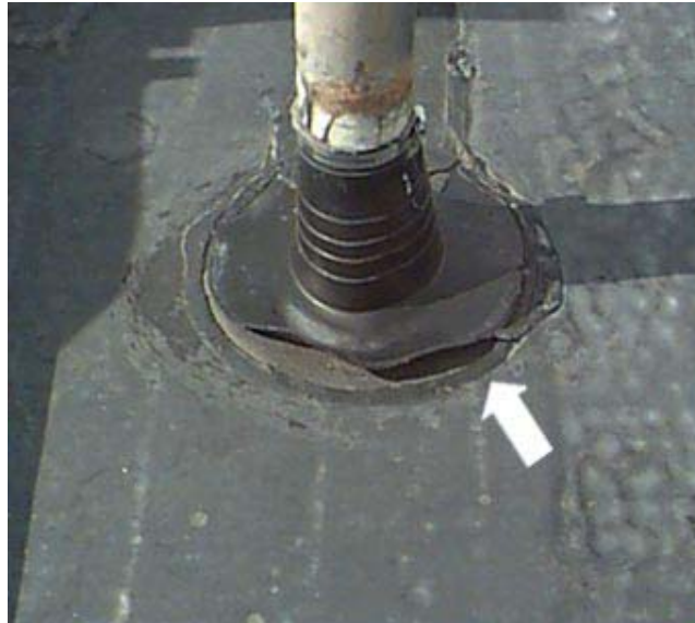
Stripping material is open. High Severity
