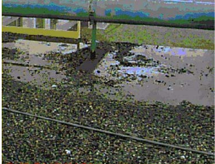
Improper location of drain. Low Severity
