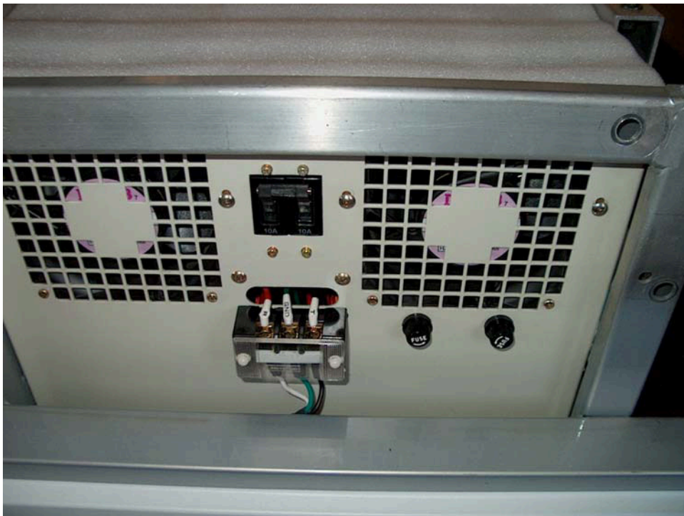
Figure A-8. Exterior of Kokam battery.
