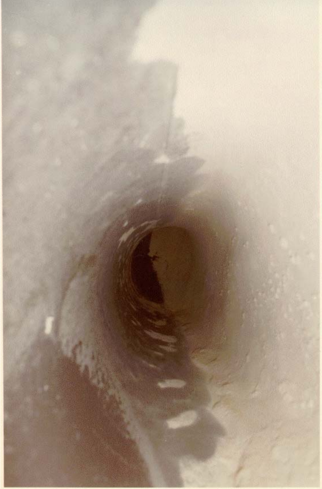
Figure A-12. Off-gas line downstream of cyclone vessel with 3 to 4 inches of calcine in the bottom of the 16-inch pipe (81-5540).
