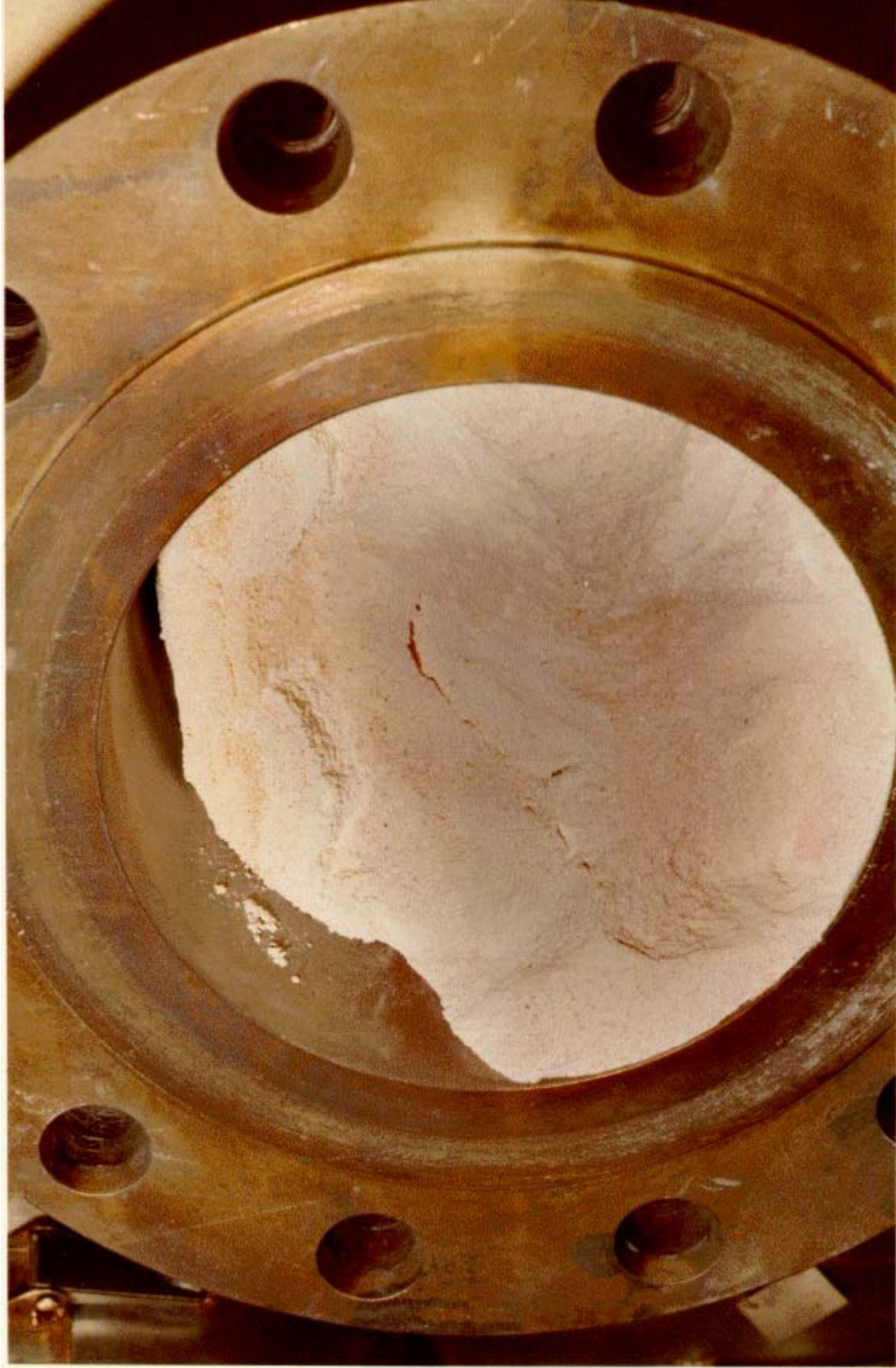
Figure A-9. Calciner east handhole (8-inch nozzle) located just above the fluidizing air distributor plate filled with calcine prior to decontamination (81-5579).
