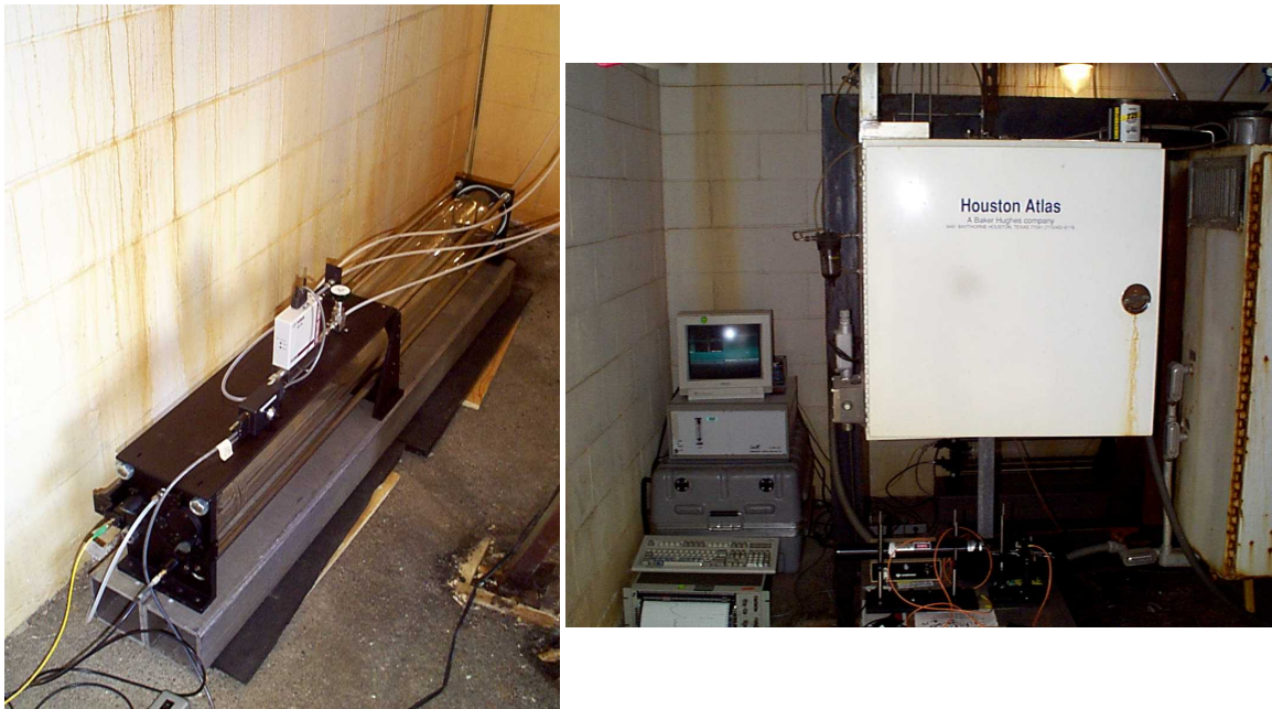
Figure 24. Multi-pass cell (left) and near-infrared spectroscopy instrumentation (right) deployed behind Houston Atlas system at NCPA Unit 1.
