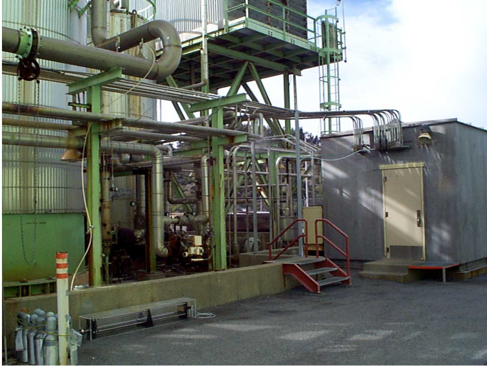
Figure 26. Stretford control room at NCPA Unit 2.
