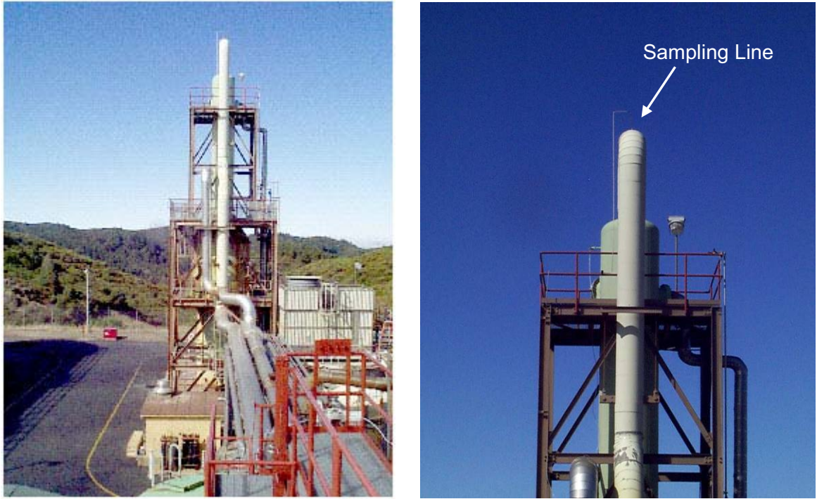
Figure 23. Overview and close-up images of treated vent gas stream sampling location.
