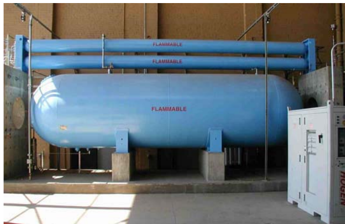
Figure 3. Low-pressure hydrogen storage tank (large, lower tank), high-pressure storage tanks (two upper tanks), and HOGEN fuel cell (right).
