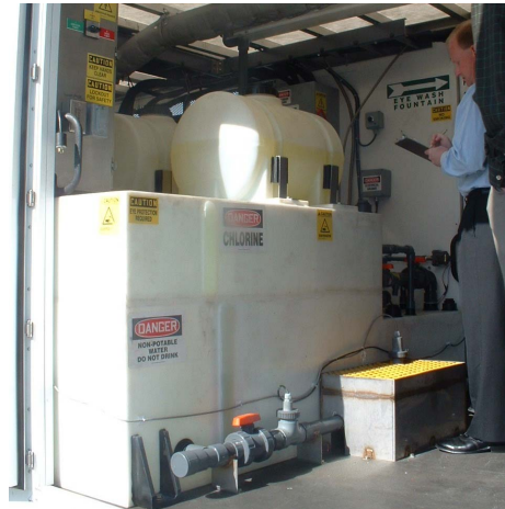
Figure 8. The on-board disinfectant chemical solution supply system tanks and other components.
