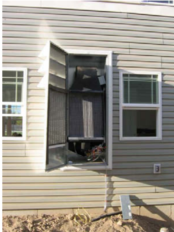
Figure 4. OASys unit installed at Magna Unit 1
