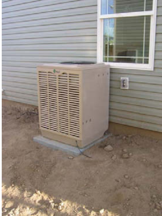
Figure 5. Freus condensing unit installed at Magna Unit 2
