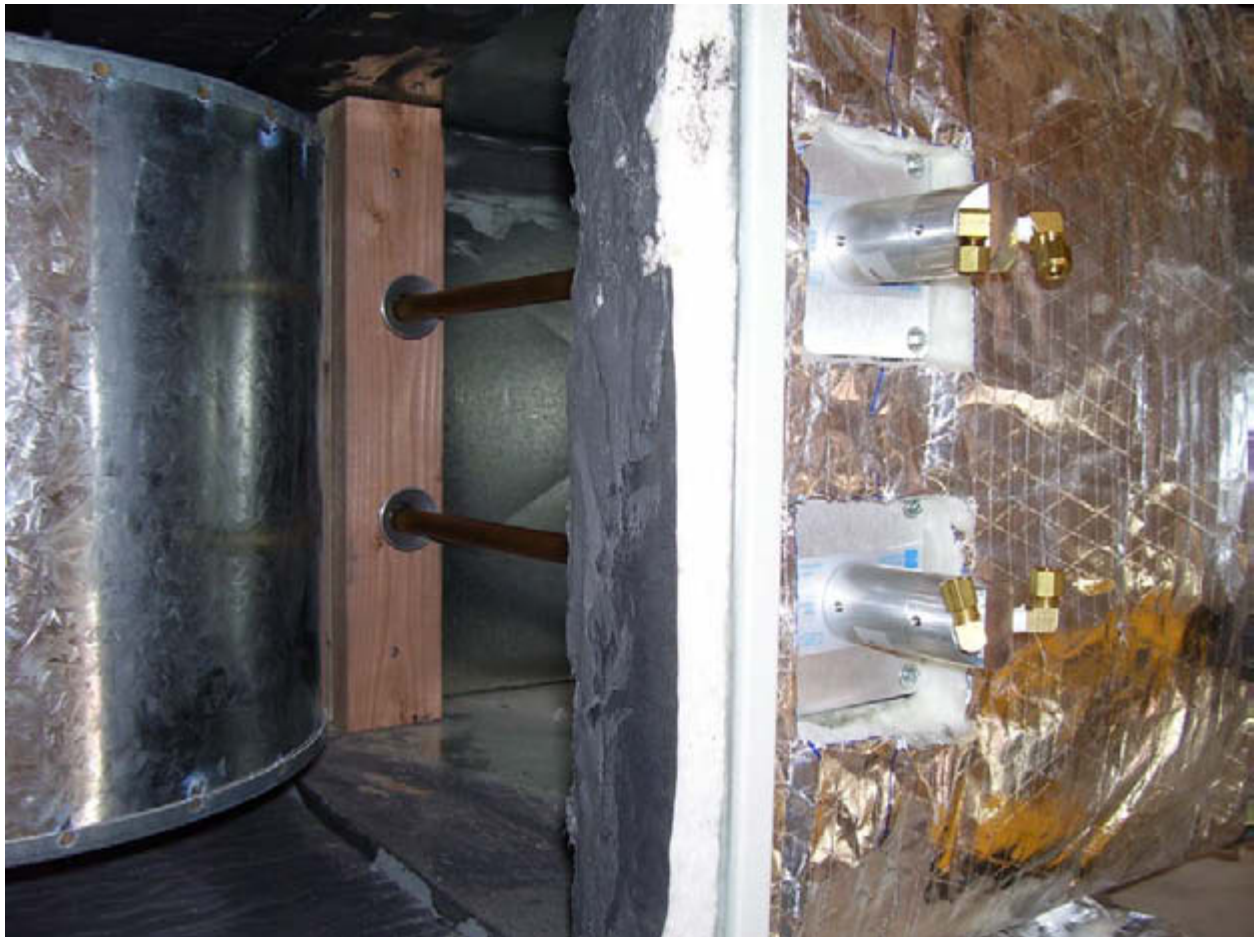
Figure 23. Pitot tube traverse airflow sensors installed at the return duct for the DiGiorgio home
