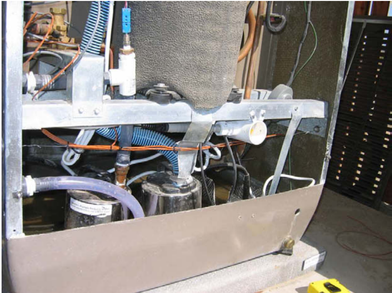
Figure 26. Thermocouple (brown wire) and Vaisala temperature and RH sensors (white PVC shield + gray sensor) installed at Freus air intake, grill removed
