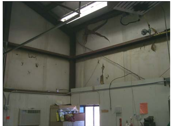
Figure 19 (PH0006) Northeast corner where a dent was present.
