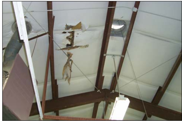
Figure 26 (PH0007) The vents were found open.
