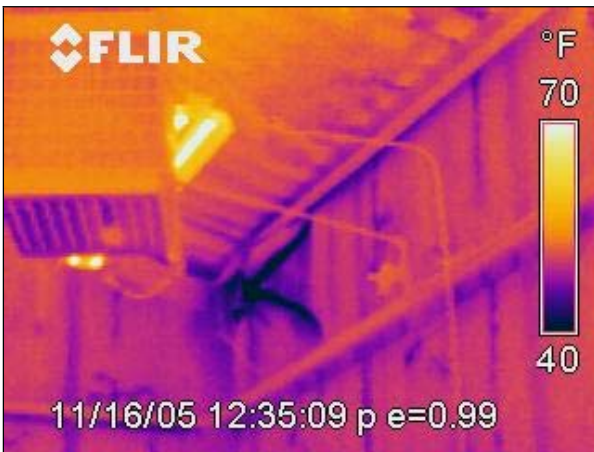
Figure 18 (IR0005) Northeast corner where a dent was present.
