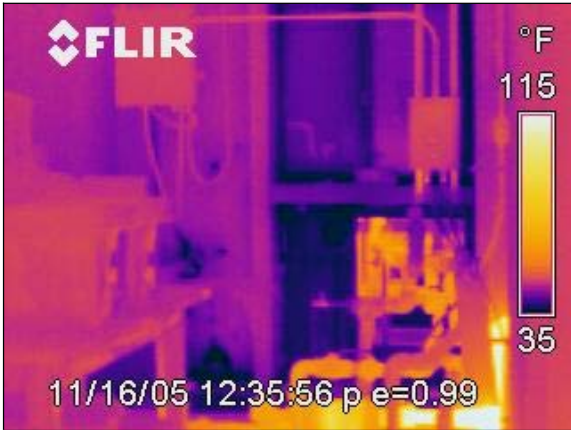
Figure 20 (IR0006) Where hot water comes into the building.
