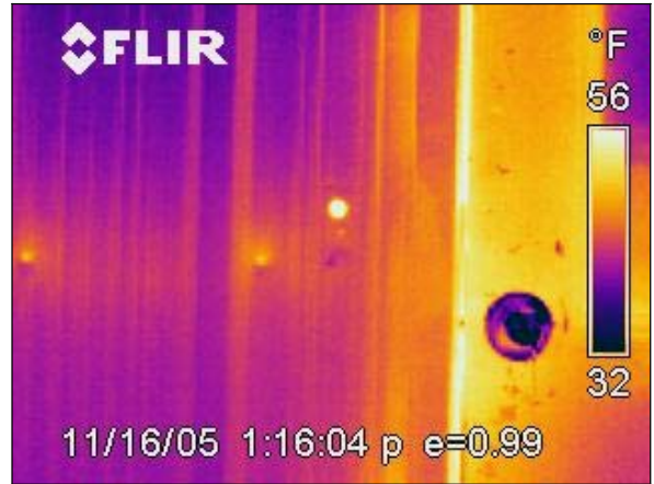
Figure 8 (IR0010) Hole where door bell use to be on the ESSH building.
