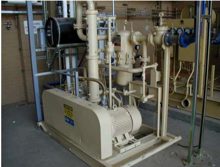
Figure 3.1. Hy-Bon - CNG boost compressor.
