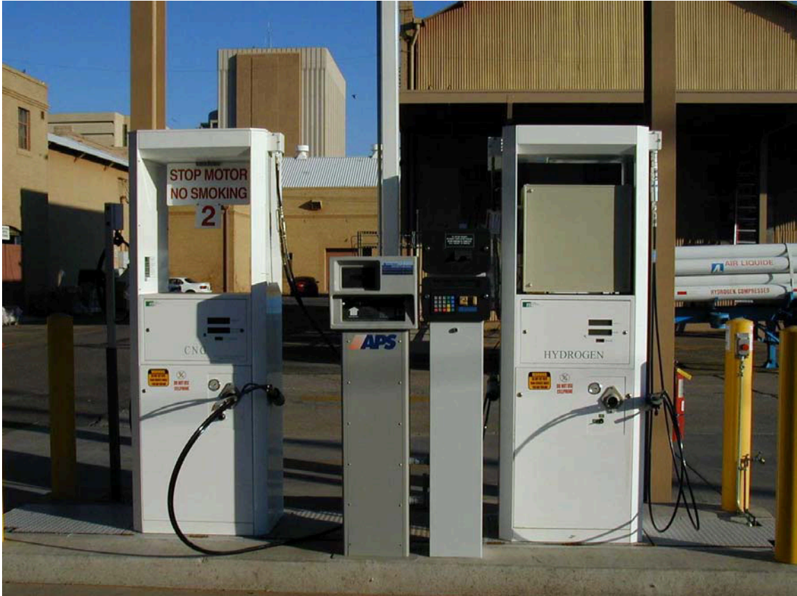
Figure 2.4. CNG only dispenser and hydrogen and CNG/hydrogen blend dispenser.
