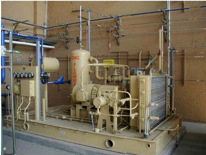
Figure 3.2. Gemini - main CNG compressor.
