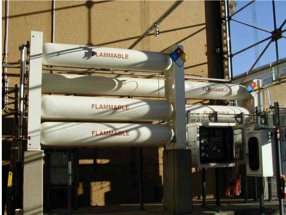
Figure 3.3. CNG storage tanks. The top tank is the high-pressure tank and the two lower tanks are the medium-pressure tanks in the near rack. The three low-pressure tanks are in the far rack.
