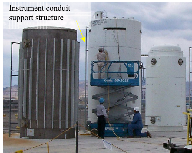
Fig. 4. Electrical conduit is visible from behind the VSC-17 cask.
