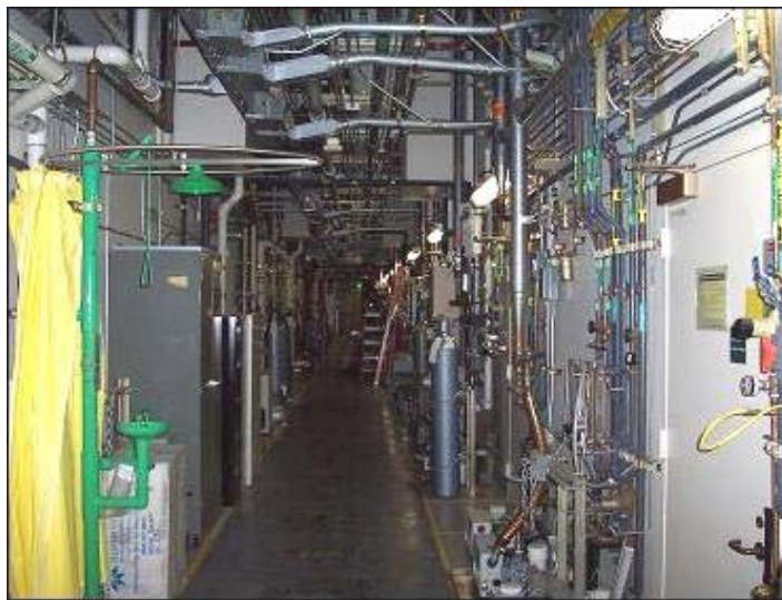
Utility corridor behind laboratories (Photo courtesy of K. Kostelnik)
