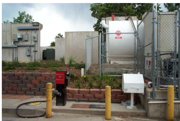
Figure 2. B20 Fueling Station
