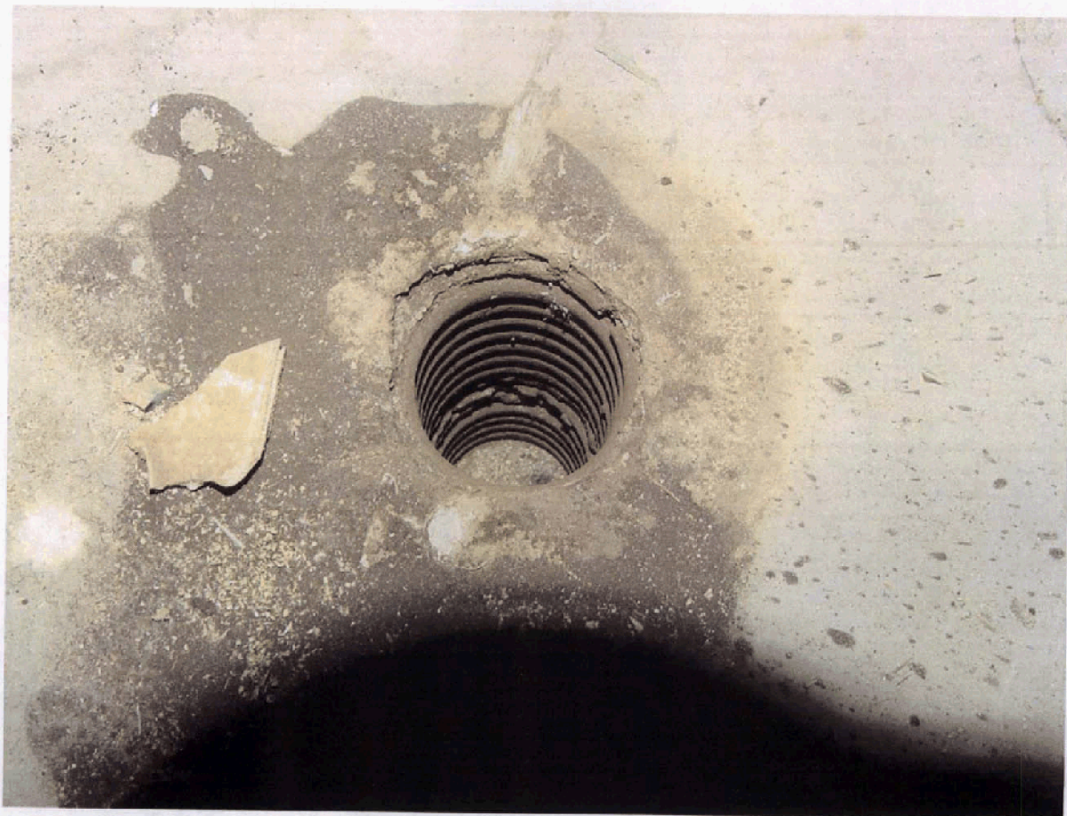
Figure 1. Typical Corroded Cask Lifting Insert Showing Broken and Missing Threads
