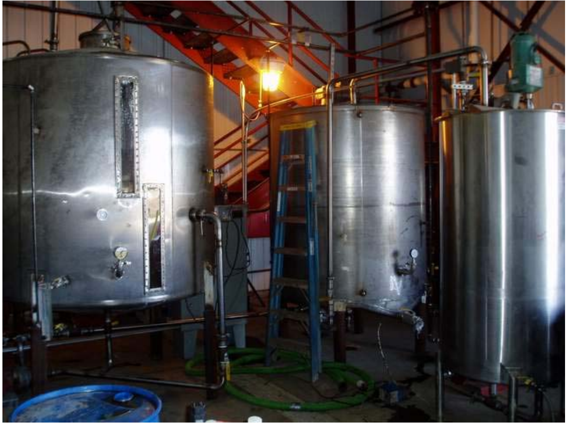
Figure 3.1.7 Completed 4500 L pilot HS/LE system
