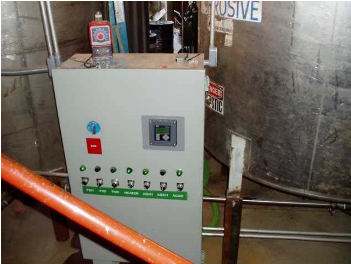
Figure 3.1.8. Control Panel for Pilot system
