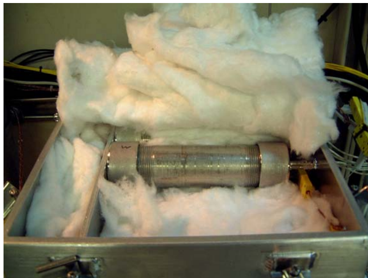
Figure 7. Heater assembly installed in insulated pipe nipple. Six of these are installed in the insulated box.
