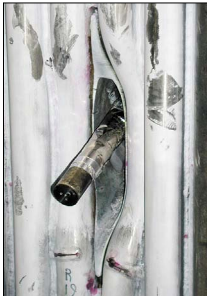
Fig. 30. Camera probe inserted through primary air port opening during a shutdown; it records activities on the fireside of the primary air port.
