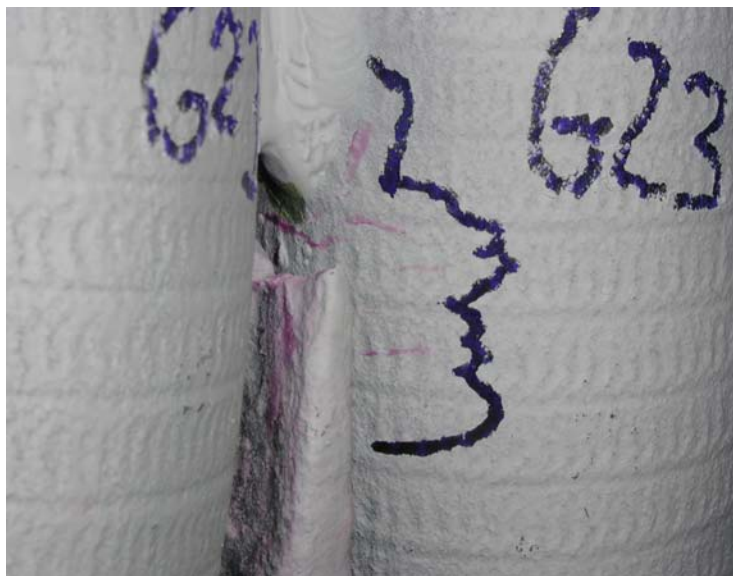
Fig. 115. Photograph showing tube and membrane cracks in upper crotch of a primary air port (Port B) comprised of GBEST/CS composite tubes installed in Boiler 10 after 36 months service.
