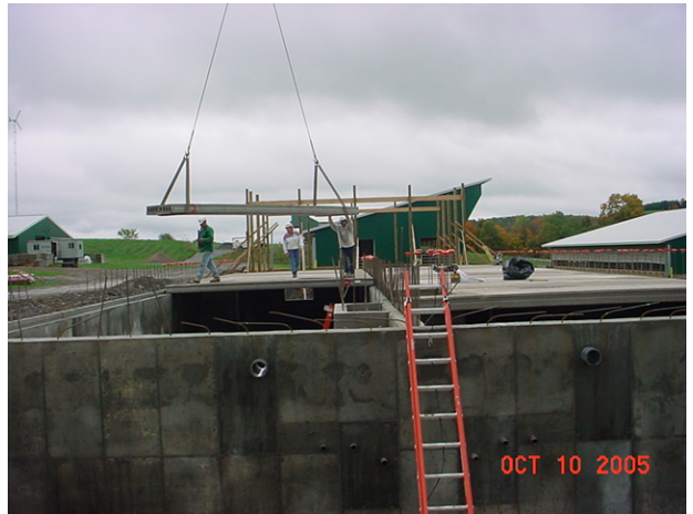
Figure 10. Laying of a pre-cast concrete plank on the NE chamber of the digester (picture taken on October 10, 2005, from near the NW wall of the digester, i.e., influent side).
