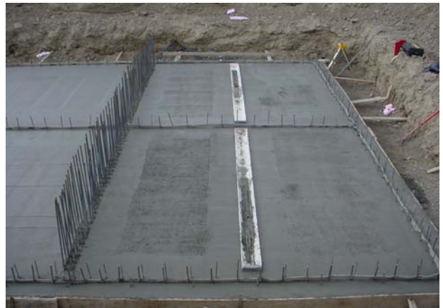
Figure 4. Closeup of the grit chamber section (15.3' long) of the tank showing \frac{1}{2} of the 4" Sch. 80 bottom of the chamber (picture taken on August 23, 2005).
