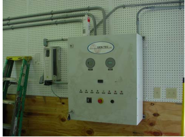
Figure 32. View of a control panel inside the equipment building (picture taken on July 20, 2006).
