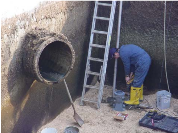
Figure 47. View of NW wall of the subdivided 3-day storage tank as the pump is being installed (picture taken on November 28, 2006).
