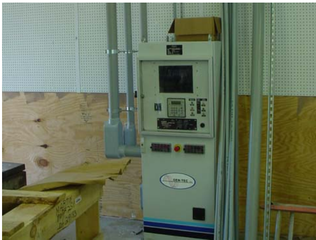
Figure 33. View of the installed system controller inside the equipment building (picture taken on July 20, 2006).
