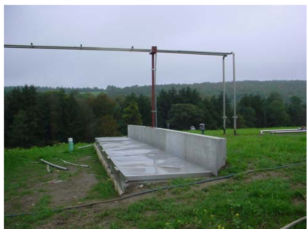
Figure 42. View of the effluent side of the digester showing the installed aluminum covers (picture taken on September 15, 2006).
