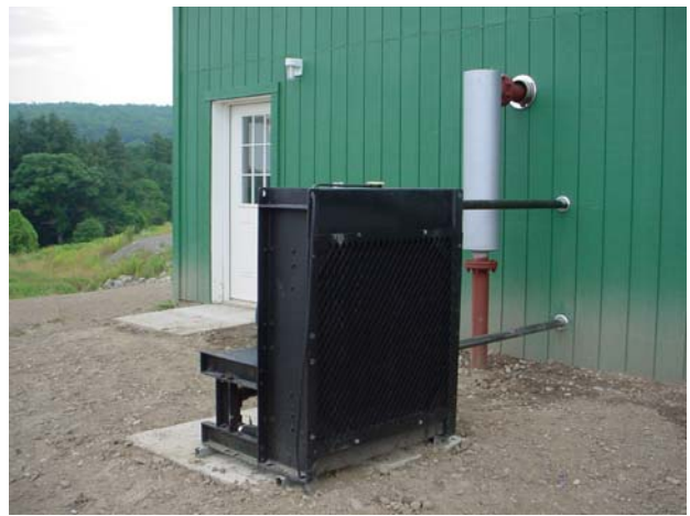
Figure 34. View of the ICE-exhaust connected to a muffler mounted on the outside of the SE wall of the equipment building (picture taken on August 7, 2006).
