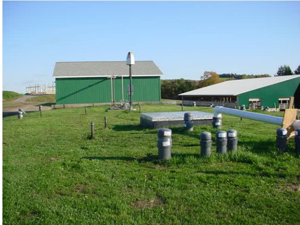
Figure 37. View of the digester and equipment building (picture taken on October 2, 2006).
