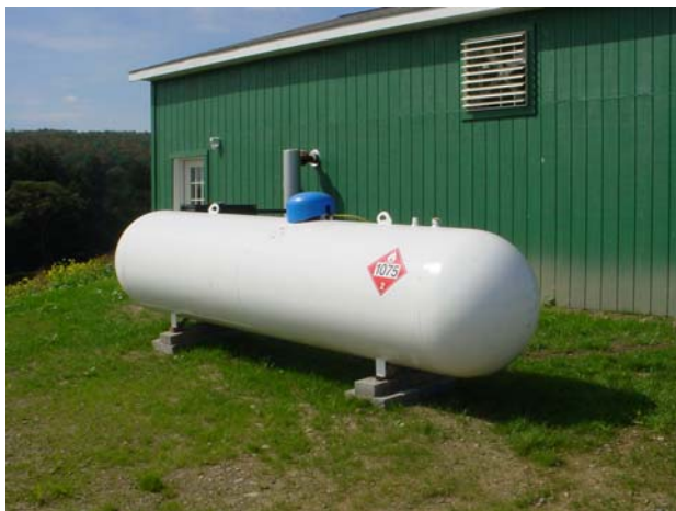
Figure 39. View of the propane tank installed near the SE side of the equipment building (picture taken on September 22, 2006).
