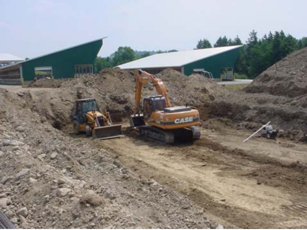
Figure 1. Site excavation for the foundation of the dual-chamber digester tank (picture taken on August 9, 2005).
