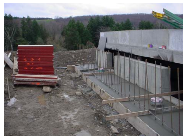
Figure 17. View of the SE wall of the digester showing the slab for the outlet bay and the openings for the cover plates on the effluent side (picture taken on November 11, 2005).
