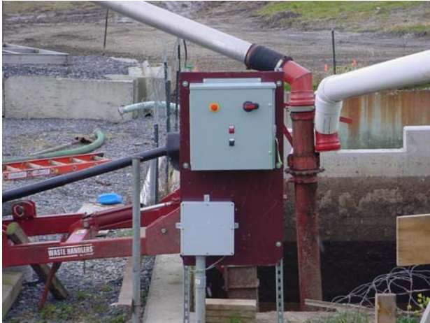
Figure 45. View of the installed pump control panel taken on November 3, 2006.
