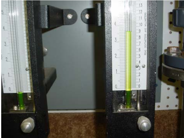
Figure 43. View of the manometer showing the biogas pressure in the SW side of the digester (picture was taken on November 4, 2006).
