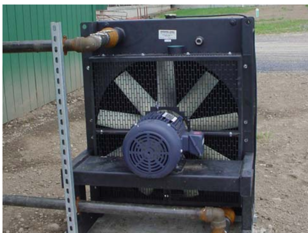
Figure 35. View of the installed radiator on a pad SE of the equipment building (picture taken on August 7, 2006).
