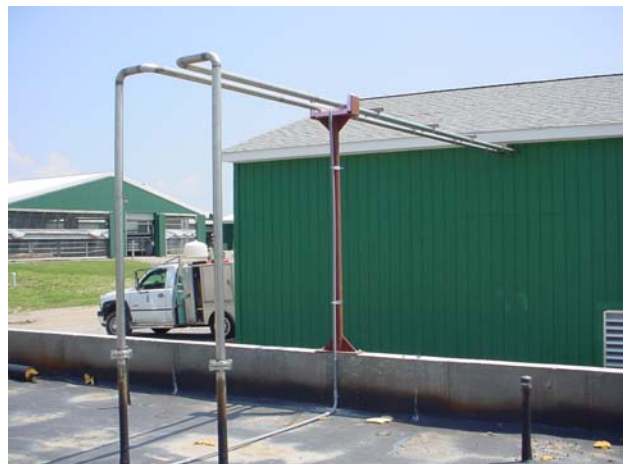
Figure 30. View of the installed gas lines from the digester to the equipment building (picture taken on July 20, 2006).
