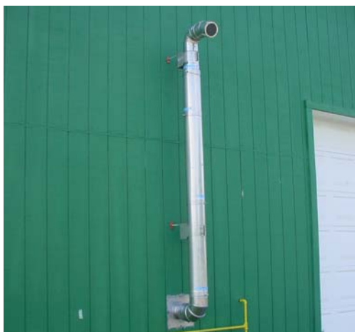
Figure 41. View of the installed boiler exhaust which was anchored to the northeast side of the equipment building (picture taken on September 22, 2006).
