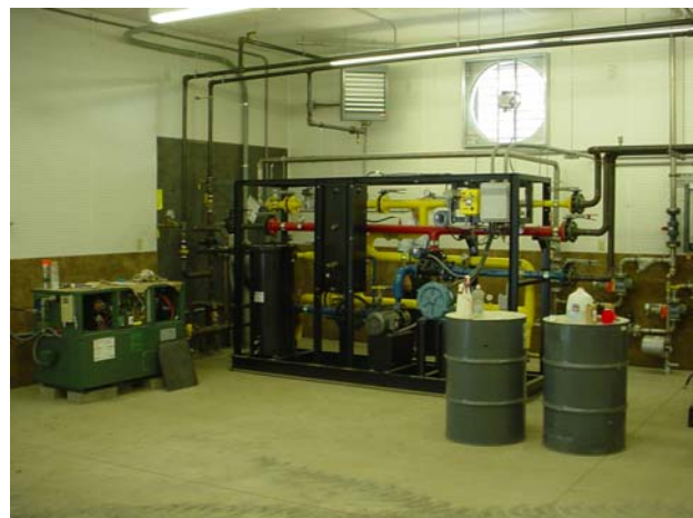
Figure 40. View of the installed boiler (left) and thermal skid (picture taken inside the equipment building on September 22, 2006).
