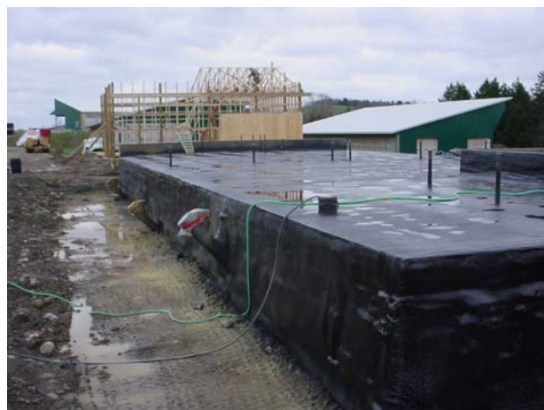
Figure 16. View of the NE side of the digester after the top and the outside walls were insulated with a layer of 2.5" of polyurethane (picture taken on November 11, 2005).
