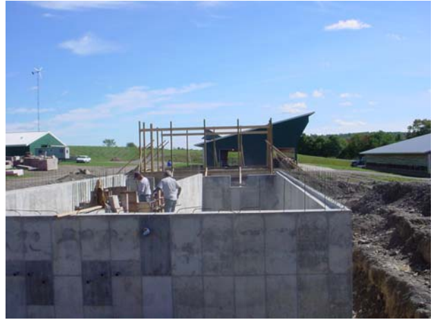
Figure 8. Completed walls of the digester showing both the influent (near side of the picture) and effluent sides of the digester (picture taken on September 30, 2005).
