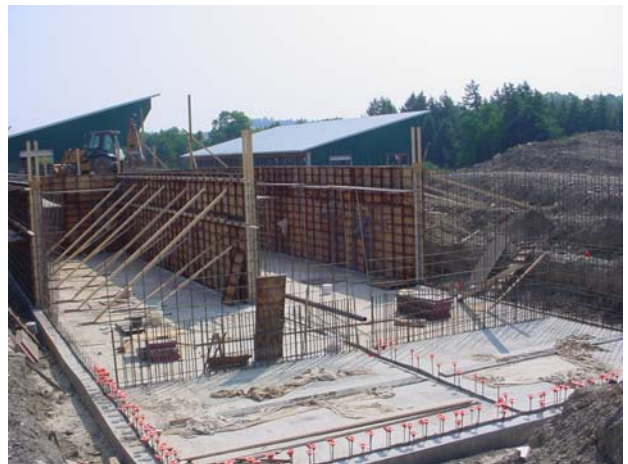
Figure 6. Completed half of the walls of the digester (picture taken from near the N-E corner on September 12, 2005).
