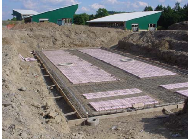
Figure 2. Form of the bottom of the tank (picture taken from near the north-east side of the tank on August 16, 2005).
