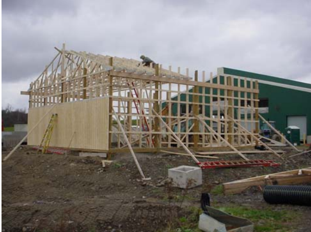
Figure 19. Completed frame of the combined heat and power (CHP) building (picture taken on November 11, 2005, showing a part of the siding of the SW side of the CHP).
