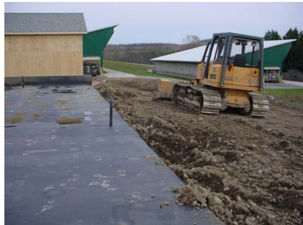
Figure 22. View of the completed backfill on the SW side of the digester (picture taken on November 21, 2005).
