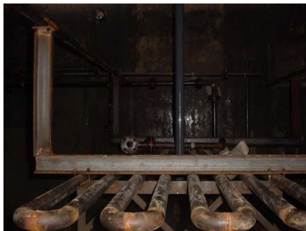
Figure 14. View of the heat exchanger inside the NE grit chamber (picture taken on October 14, 2005, showing one of the two access tubes that penetrate through the top).
