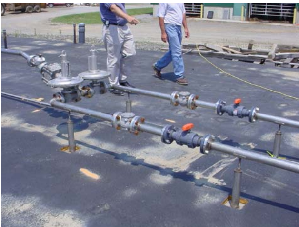
Figure 29. View of the installed gas lines from the two chambers of the digester to the flare (picture taken on July 20, 2006).
