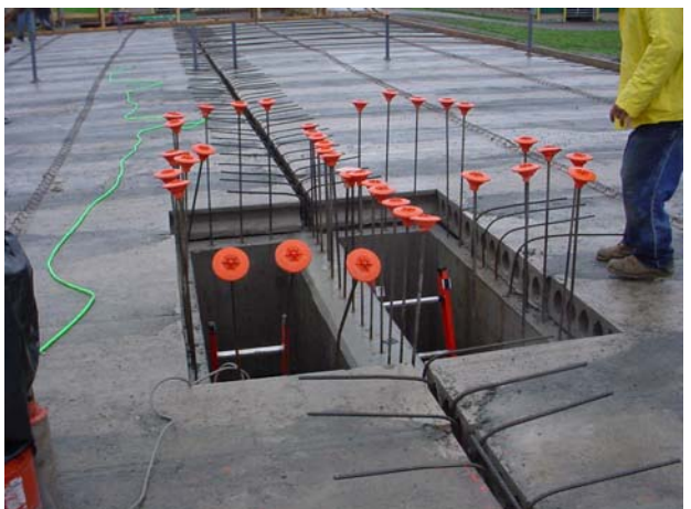
Figure 12. View of the access ports section of the digester top before pouring the 4" concrete top coat (picture taken on October 14, 2005).
