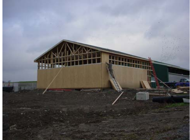
Figure 20. View of the back and the SW side of the CHP building (picture taken on November 17, 2005).
