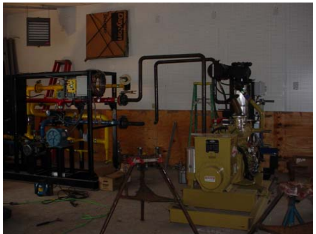
Figure 28. View of the partially connected thermal and ICE/generator skids inside the CHP building (picture taken on May 23, 2006).
