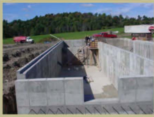
Close-up of one of the chambers from the effluent side of the digester (9/30/05)
