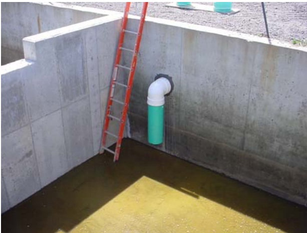
Figure 27. View of the S-W wall of the effluent compartment of the storage tank showing the outlet location of the effluent pipe from the digester (picture taken on May 2, 2006).
