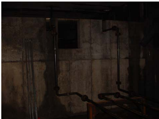
Figure 13. View of the maintenance heat loop near the wall of NE grit chamber (picture taken on October 14, 2005, inside the NE chamber of the digester).
