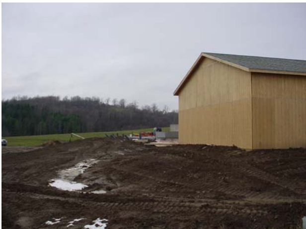
Figure 23. A view of the back (SW) side of the CHP building after the backfill was completed (picture taken on November 28, 2005).
