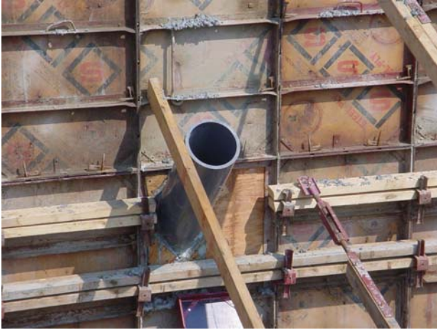
Figure 7. Form on the south-west wall of the digester showing the location of one of three wall penetrations on each side of the tank (picture taken on September 12, 2005).
