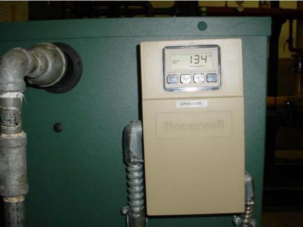
Figure 44. View of the thermostat on the boiler showing a setting of 134°F (picture was taken on November 4, 2006).
