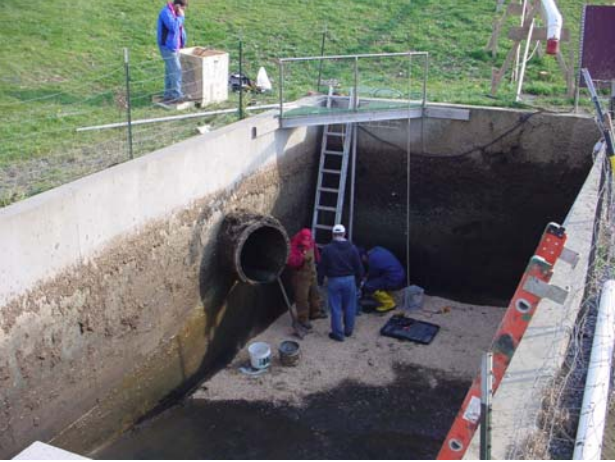
Figure 48. Another view of NW chamber of the 3-day storage tank as the pump is being installed (picture taken on November 28, 2006).
