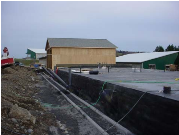
Figure 21. View of the insulated pipes that connect the CHP to the maintenance loops and heat exchangers (picture of the NE side of the digester taken on November 21, 2005).
