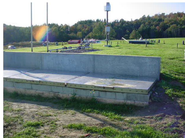
Figure 36. View of the effluent side of the digester (picture taken on October 2, 2006).
