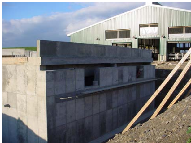
Figure 15. View of the SE wall of the digester (the effluent side of the tank) after the 4" concrete top coat was poured (picture taken on October 20, 2005).
