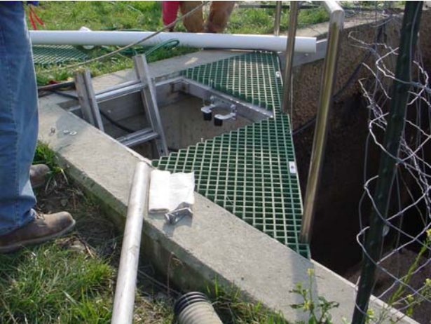
Figure 46. View of NW corner of the subdivided 3-day storage tank in preparation for the installation of the electric pump (picture taken on November 28, 2006).
