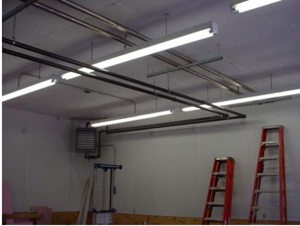
Figure 31. Inside view of the equipment building showing the two stainless gas lines from the digester and hot water lines to one of the heaters (picture taken on July 20, 2006).
