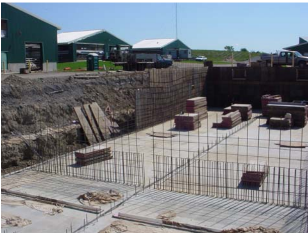
Figure 5. Preparation of form of the outside walls of the digester (picture taken from the near N-W corner of the tank on September 6, 2005).
