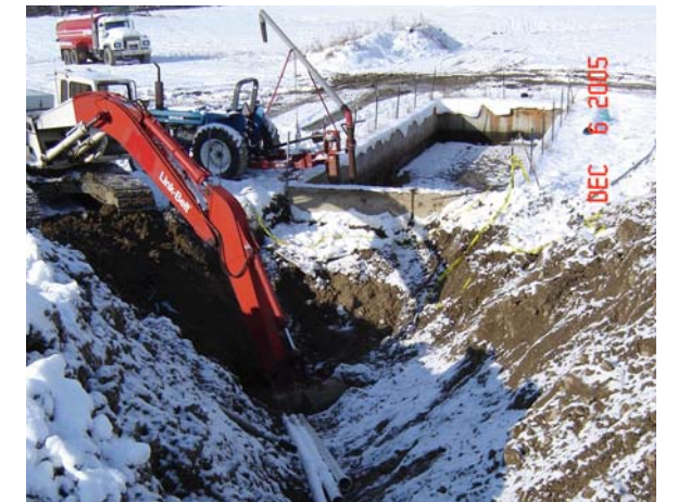
Figure 24. View of the 4" influent pipe to the digester (picture taken on December 6 th showing the pipe's location in relation to the SE side of the existing manure storage tank).
