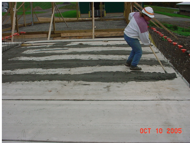
Figure 11. Sealing of the top of the planks covering the NE chamber of the digester (picture taken on October 10, 2005).
