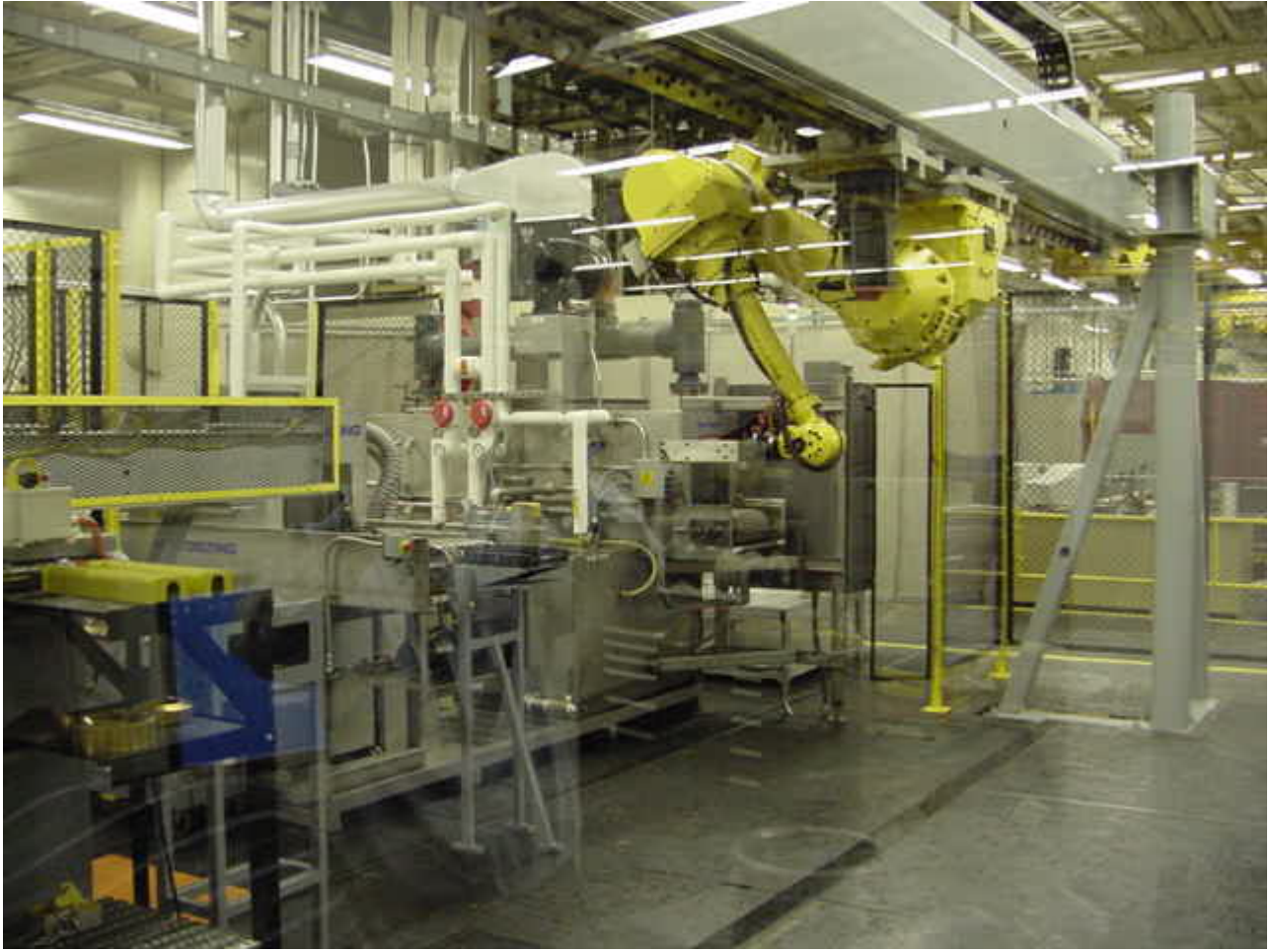
Figure 1-5 Photograph of the Thermal Treatment Cell
