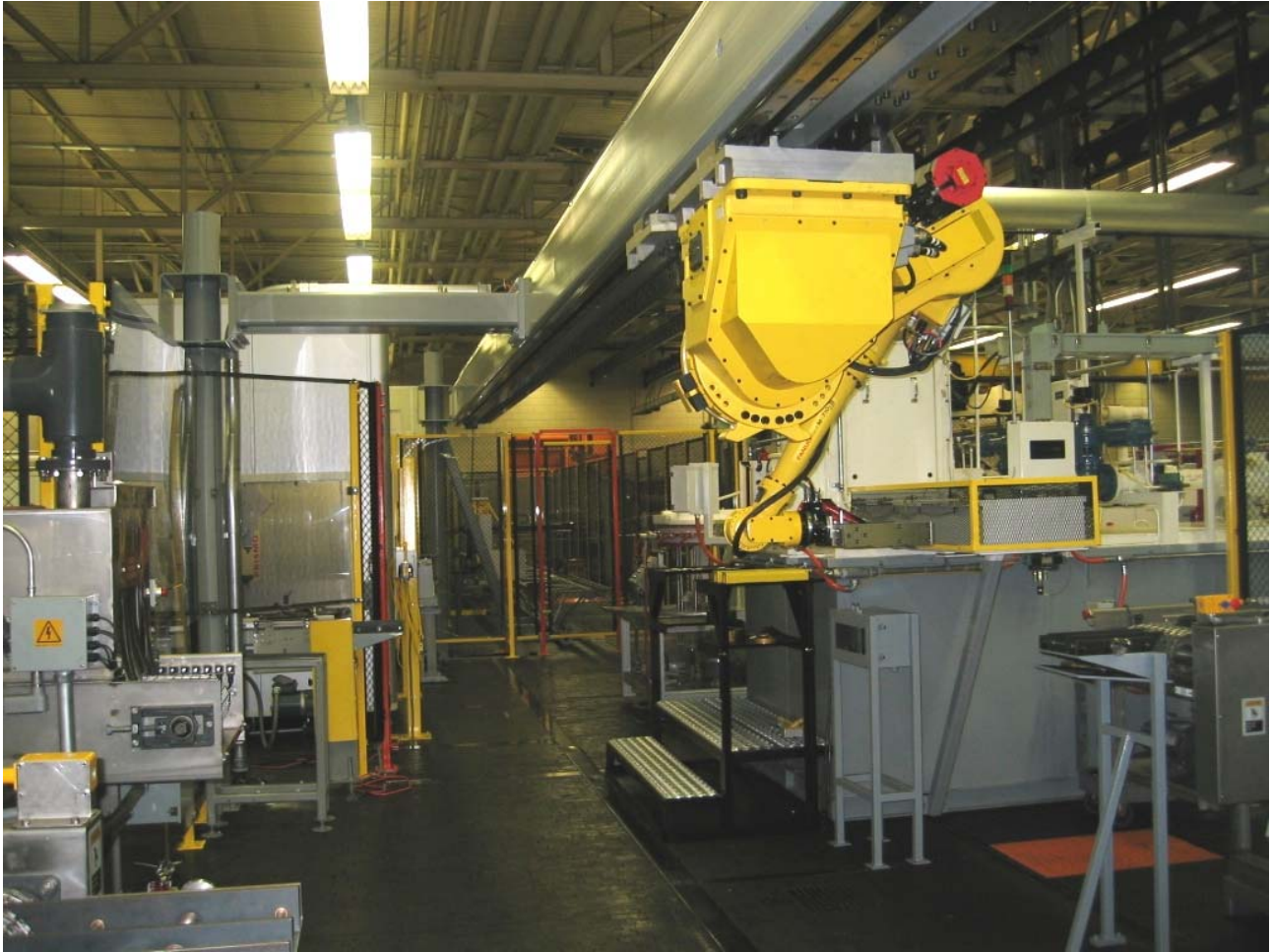
Figure 1-4 Photograph of the Thermal Treatment Cell
