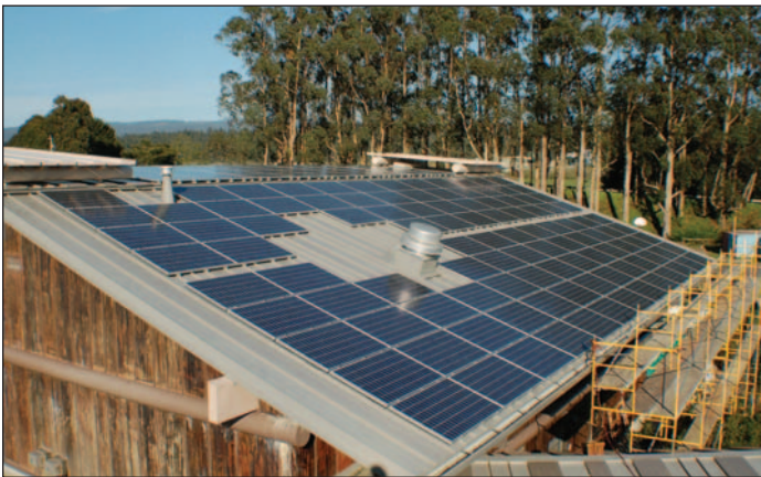
Solar panels atop the maintenance wing of the UIHS facility. Photo courtesy of UIHS.
