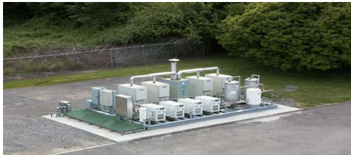
4 Capstone 30 kW Microturbines with Central Heat Recovery
