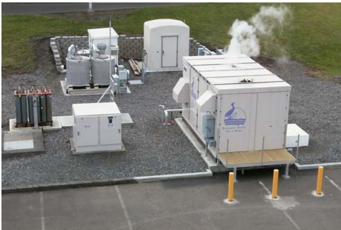
CBWTP 200kW Fuel Cell
