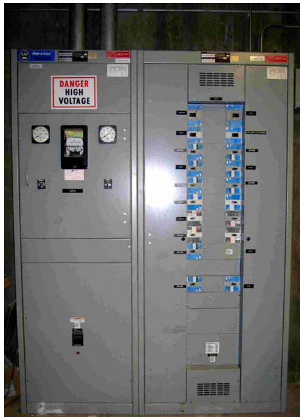
Figure 4.2. Building B - Distribution Panel with Three-Phase Lighting Riser Logger Installed in Right-Hand Compartment
