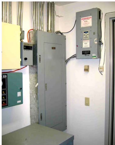
Figure 3.1. End Use Metering Logger. The box to the right of the control panel is one of two end use metering loggers used to measure current, power, and apparent power in Building A.
