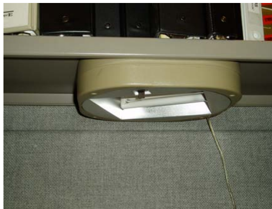
Figure 3.11. Building A Workstation Task Light
