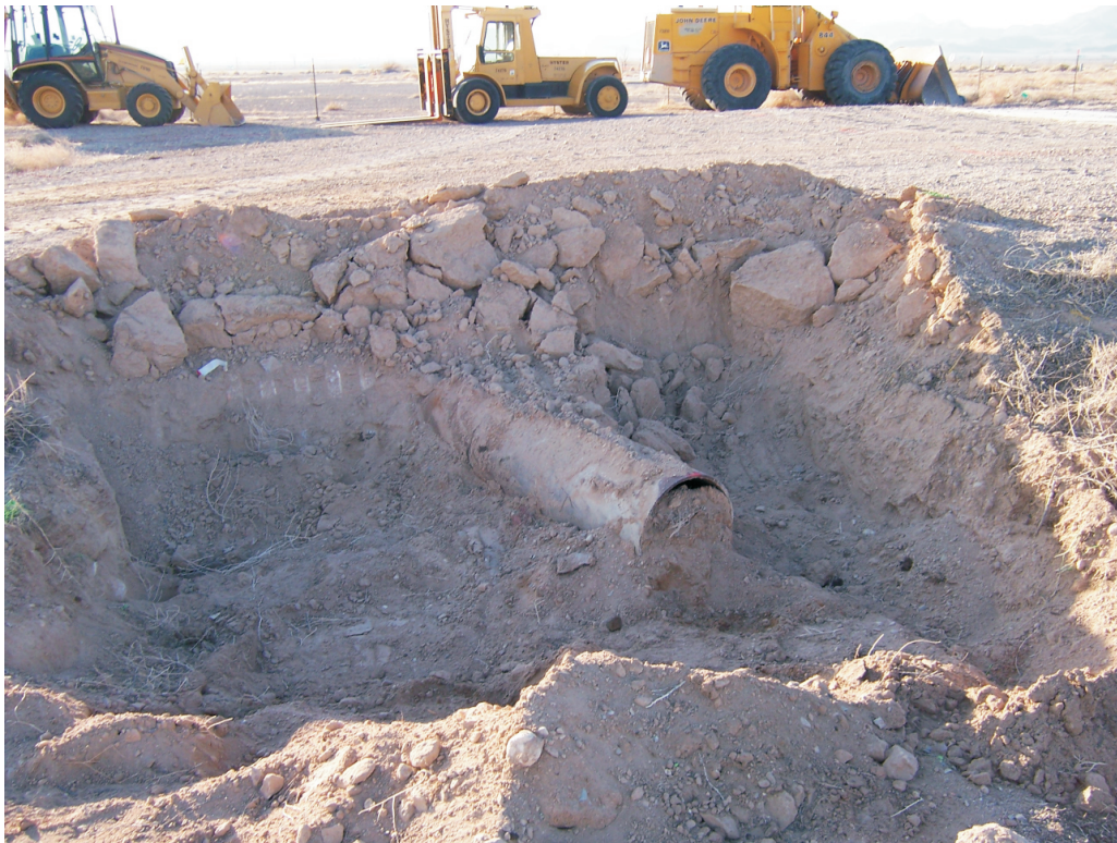
Photograph 4: Drum discovered during excavation (01/11/2007)
