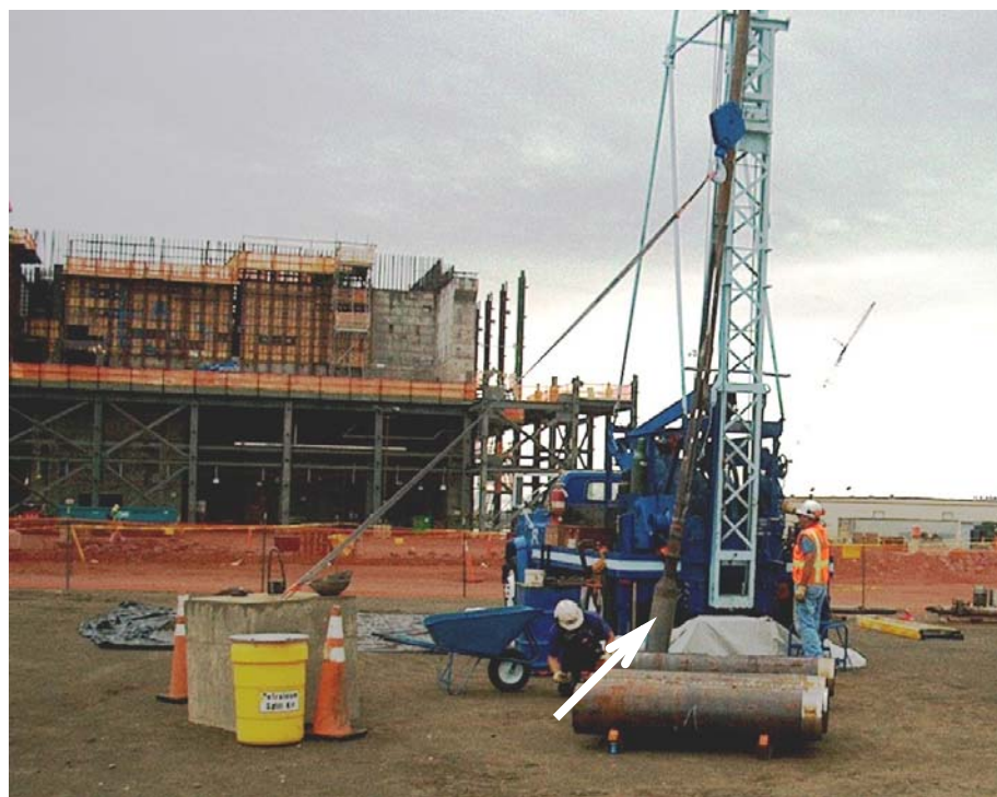
Figure 3.1. Cable-Tool Drill Used to Drill Entry Hole at Borehole C4998. The 13-3/8-in. threaded casing is seen in the foreground in front of the drive barrel (arrow), which is used to remove cuttings from the borehole as the casing is advanced.
