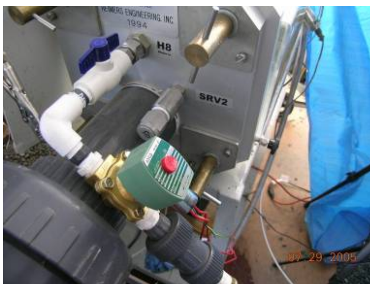
Figure 2.7. Water Inlet Valves Controlling Water Entering the Hyperbaric Chamber
