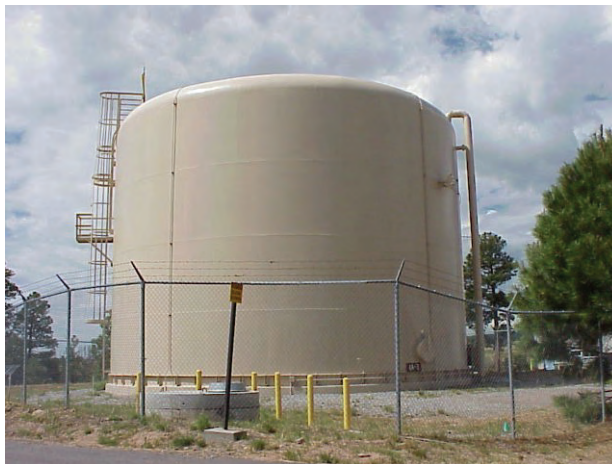
Figure 1. Air gap protection-type tank, (note the fill and overflow piping on the right).
