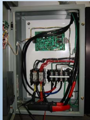
AC-DC Power Electronics
