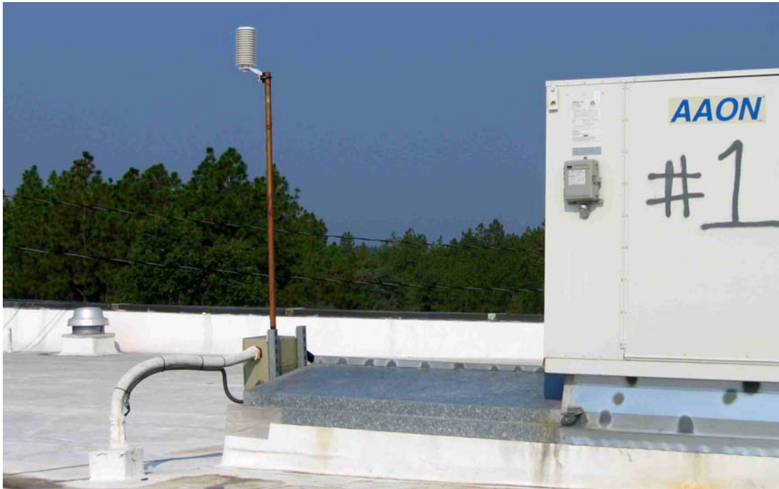
Figure F-1. Mast and radiation shield for outdoor air temperature sensor.
