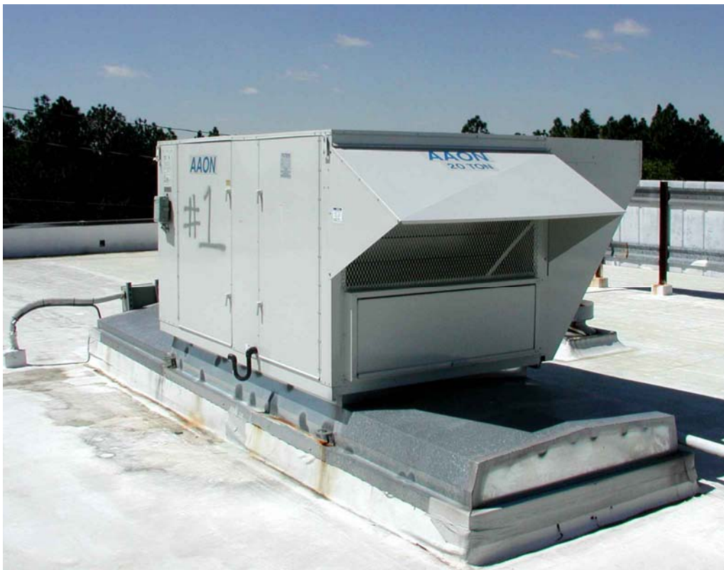
Figure 4. Fort Gordon AAON Baseline RTU
