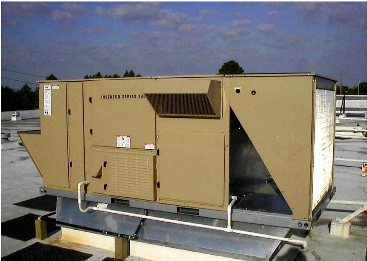
Figure 5. Fort Gordon GEG Inventor 1400 Series High-Efficiency RTU
