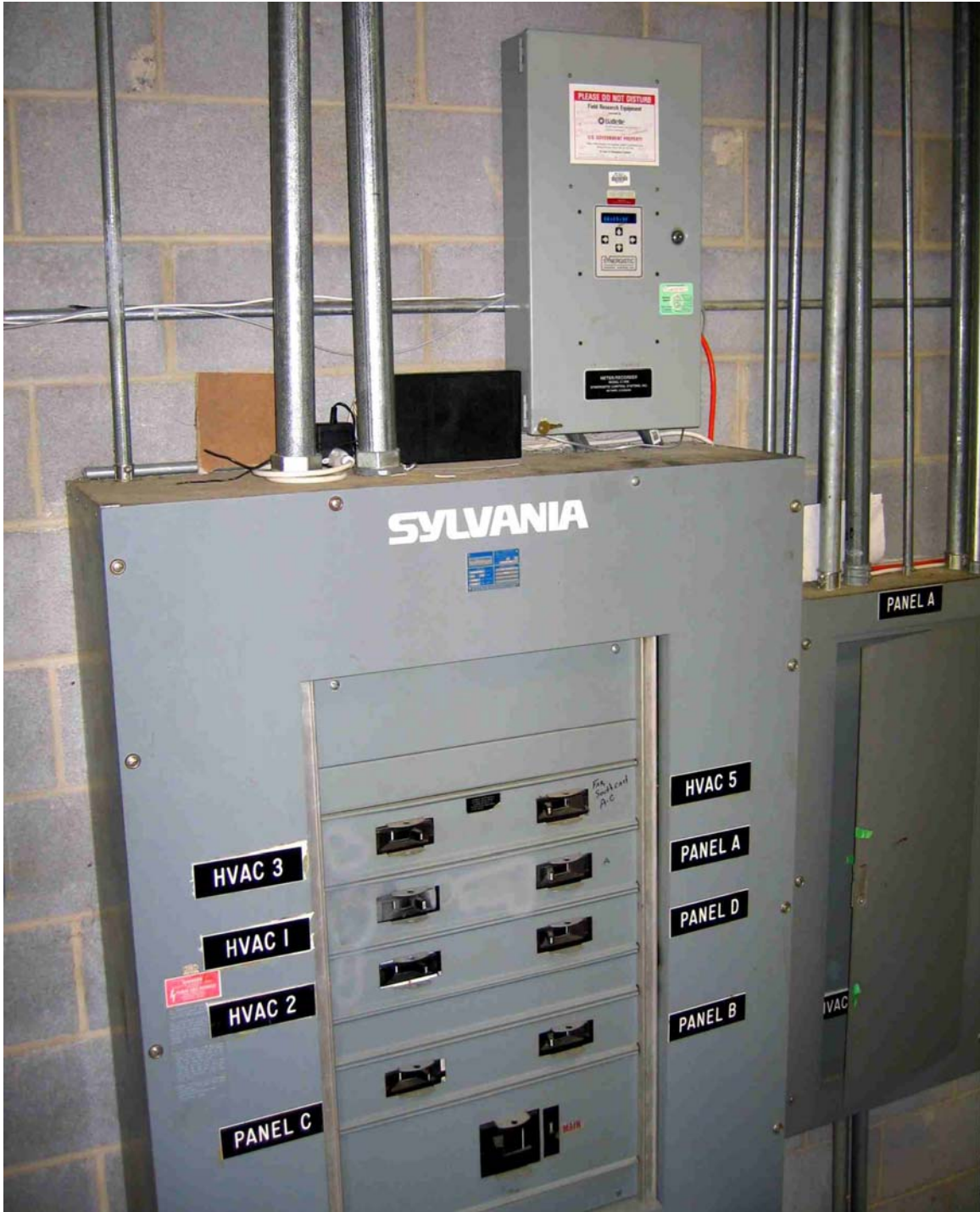
Figure 7. C180 Data Logger (upper right in photo) for Monitoring Electrical Loads
