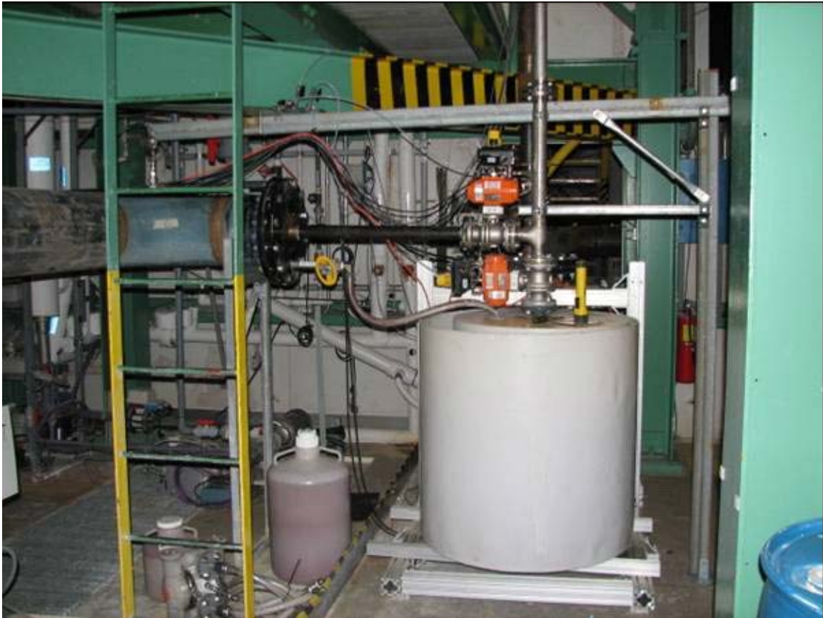
Figure 4. Photograph of Test Facility showing connection to 28 cu ft Volume
