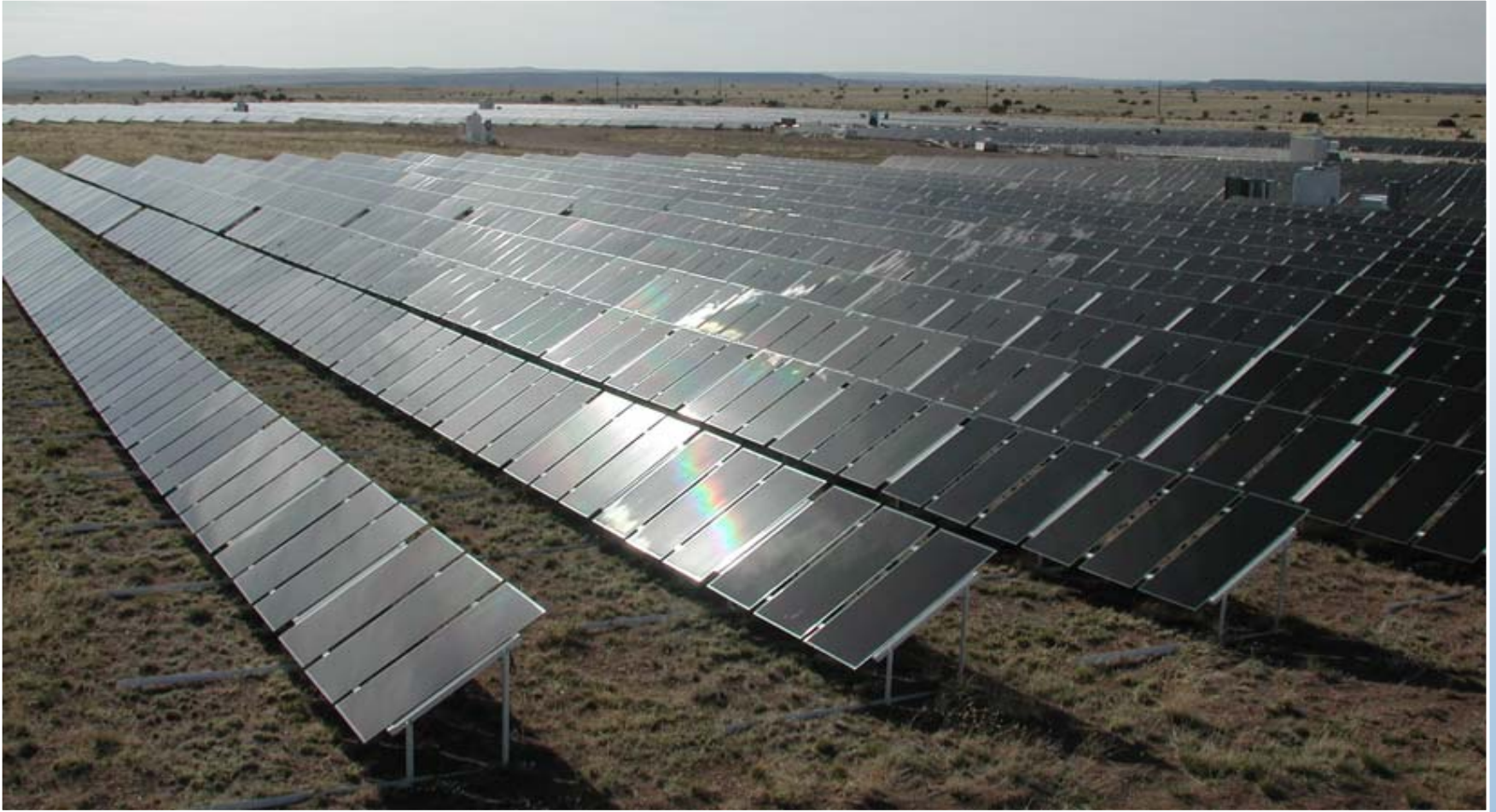
Tucson Electric/First Solar
