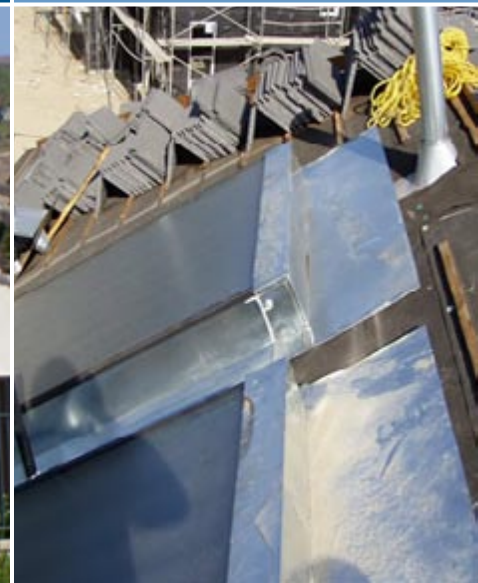
(left, right) ICS mounted directly on roof deck and integrated with mission and cement tile systems. The photos were taken at a development in Thousand Oaks, California, in 2002. Photos courtesy of John Harrison of the SRCC and FSEC.
