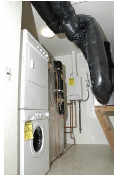
The utility room is equipped with energy-efficient appliances, the tank for the solar water heating system, and an energy recovery ventilation system. Photo courtesy of NREL.
