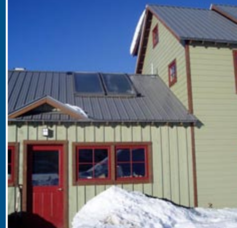
Solar collectors mounted on a standing seam roof. Photo courtesy of Leif Juell, Alternative Power Enterprises, Inc.
