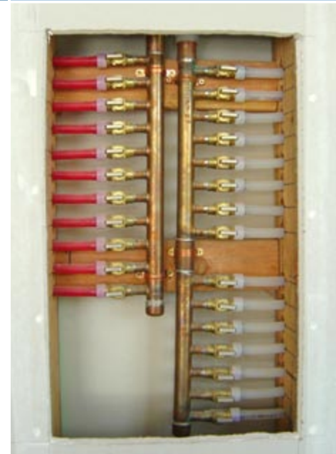
Plumbing manifold gets hot water to its destination faster.
