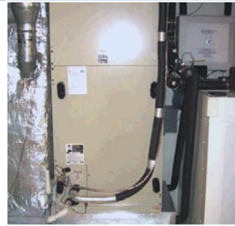
The home's A/C unit (center) and an integrated solar water and space heating system. Solar collectors provide space and water heating with backup heat provided by a tankless water heater (photo from NAHBRC).
