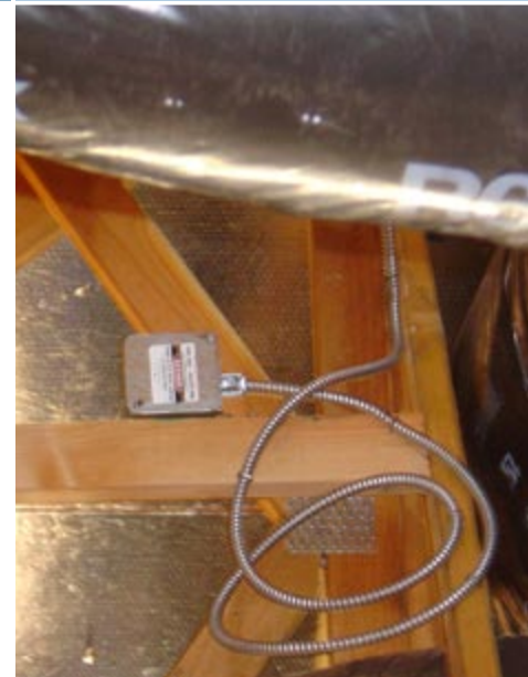
Some BIPV systems tie into a junction box that was installed during the rough-in stage of construction.
