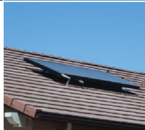
With help from Building America research, Pulte selected closed-loop, active solar water heating units.
