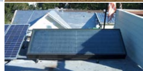
(left) This solar thermal system is ground mounted. Photo courtesy of Leif Juell, Alternative Power Enterprises, Inc.
