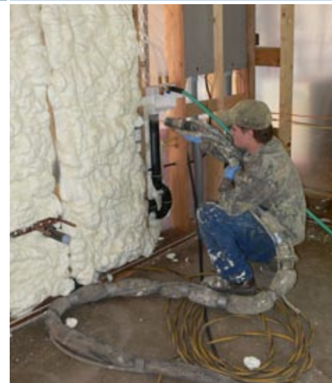
The home’s walls and ceiling received R-19 of Icynene foam, which provides excellent insulation and air sealing.
