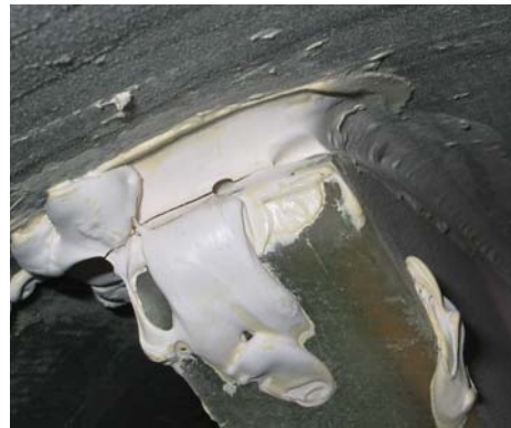
Figure 25: Crack at shear web termination on the LP surface of the BSDS blade.
