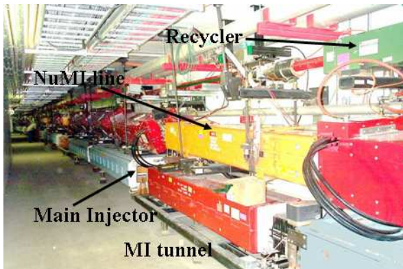
Figure 2: A photo of the Main Injector tunnel in the MI-60 region, showing the NuMI extraction line between the Main Injector at the bottom and the Recycler on top.
