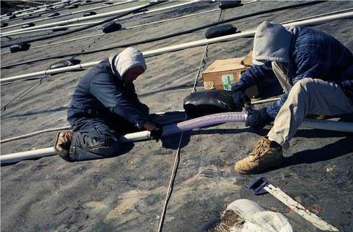
Image 25. Flexible couplers were installed to allow thermal expansion and contraction of the pipe.
