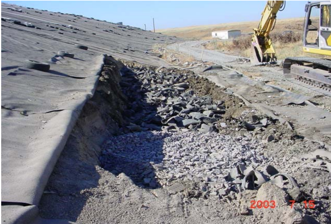
Image 43. In the area of water build up, the liner was removed and a trench was excavated and then backfilled with shredded tires and gravel
