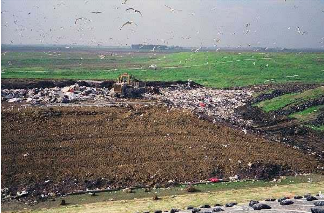
Image 3. Waste placement in valley between the west 6-acre cell and existing conventional module (left side of photo).
