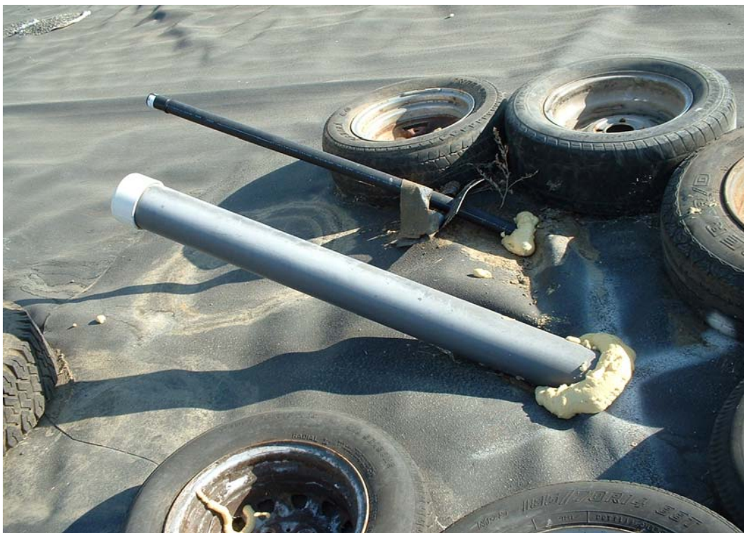
Image 50. Pipe penetrations on the west 6-acre cell were sealed with waterproof and airtight expansion foam to reduce surface emissions.
