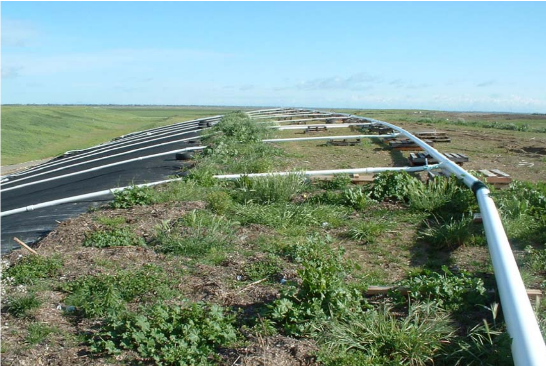
Image 26. LFG collection lines were connected to the main header line located on the top of the cell.
