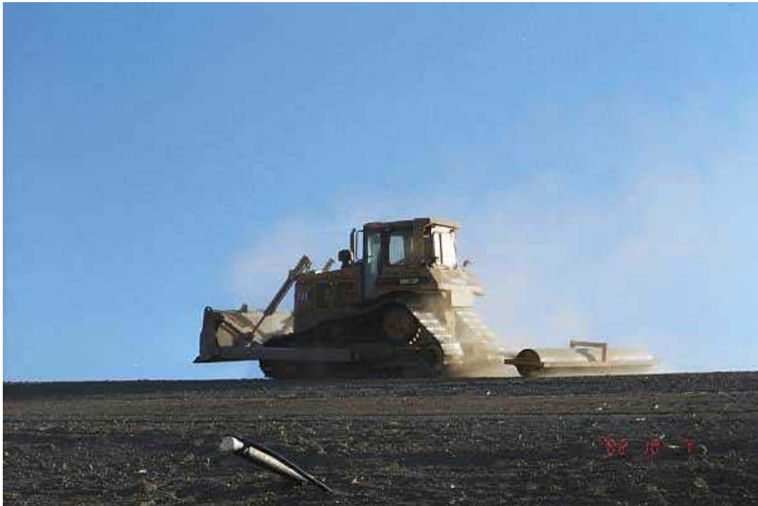
Image 28. A steel roller was used to finish the soil surface prior to liner placement
