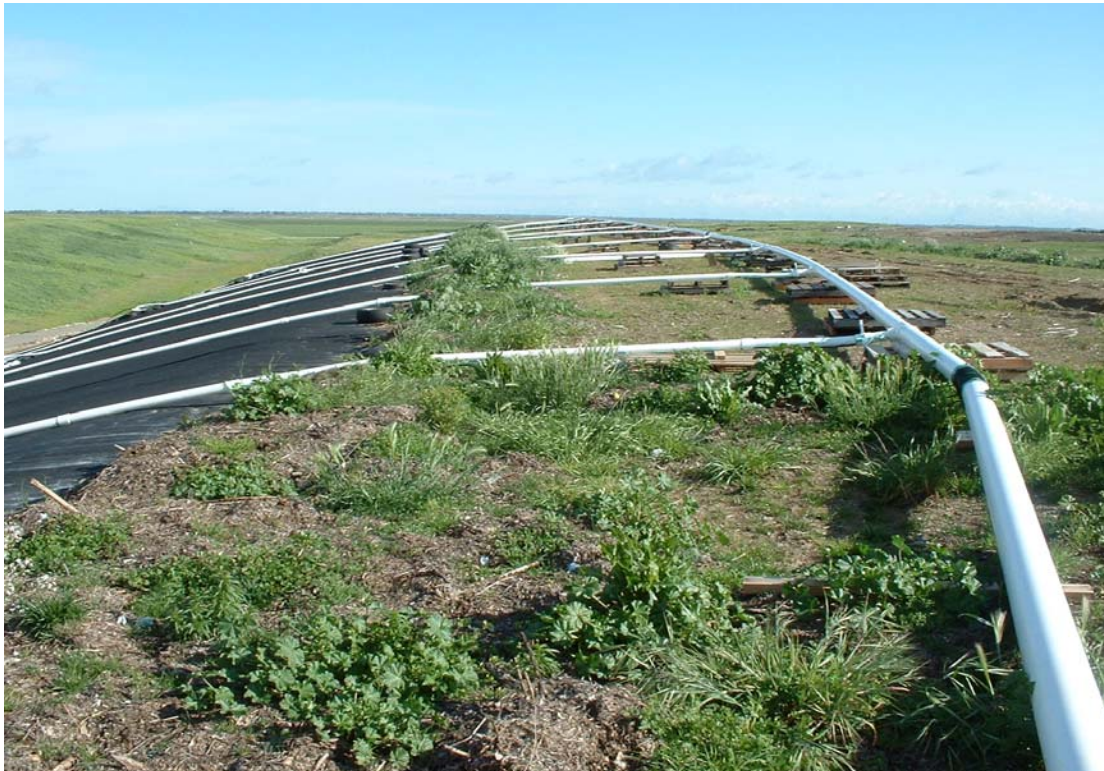
Image 3. LFG collection lines connected to the main header on the west 6-acre cell.
