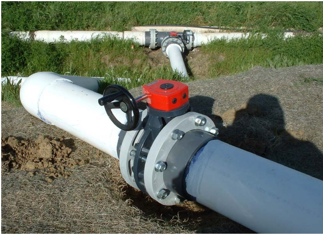
Image 27. The LFG collection header line was connected to the existing LFG collection system.
