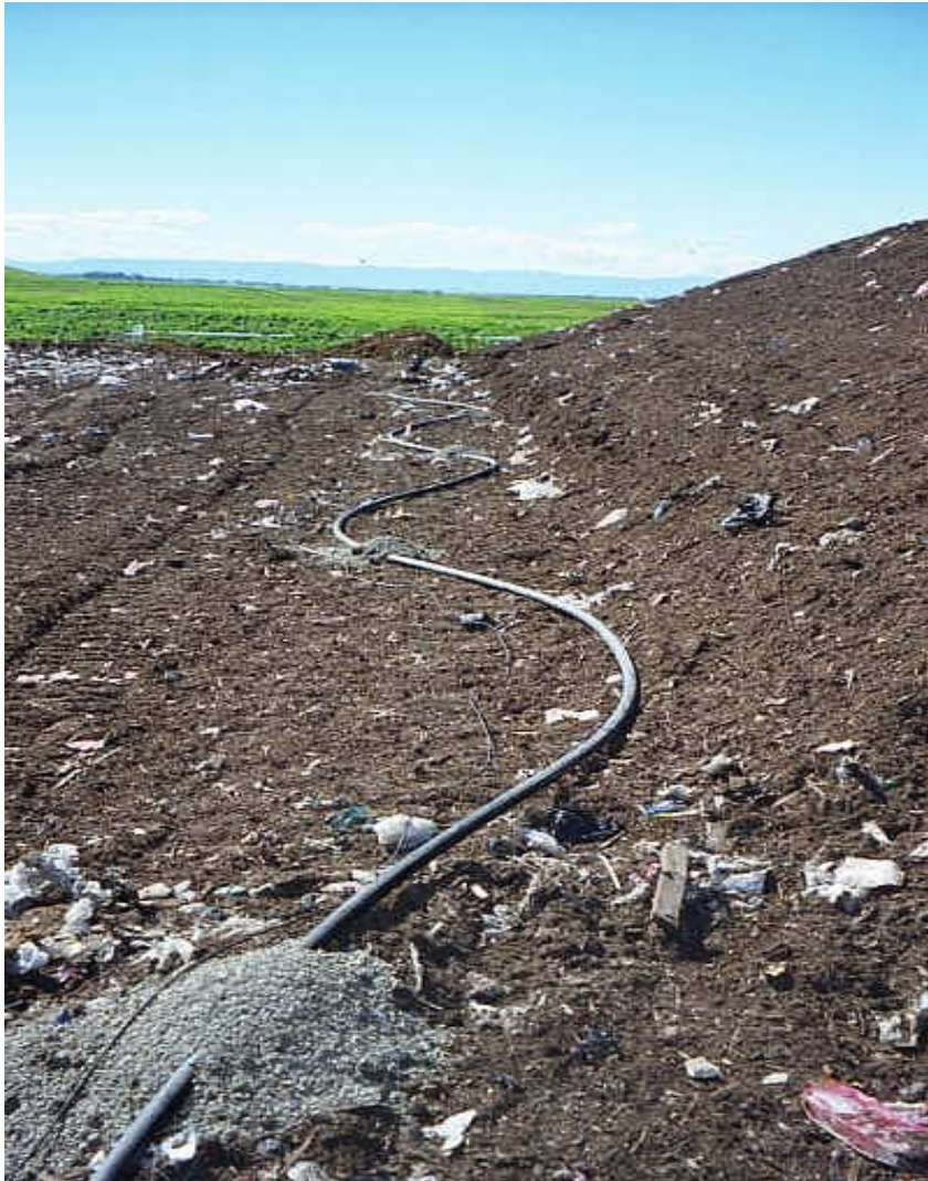
Image 17. Installation of leachate injection line, with pea gravel placed over injection holes to prevent clogging.
