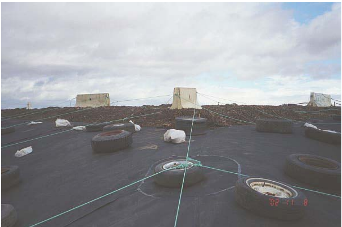
Image34. The tires were restrained from sliding down the liner by rope anchored at the top of the cell.
