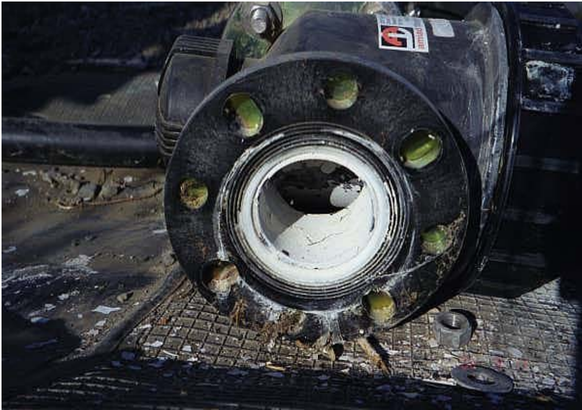
Image 41. Scale buildup on the northeast 3.5-acre leachate injection lines.
