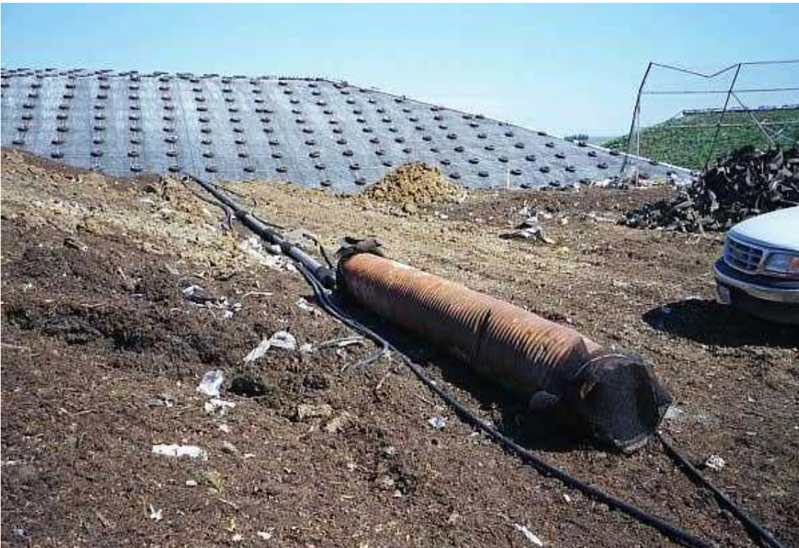
Image 22. Recycled corrugated metal pipe utilized for gas collection piping.
