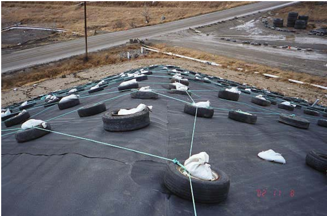
Image 35. Sandbags were placed at each tire location for additional weight to prevent wind up-lift of the liner.
