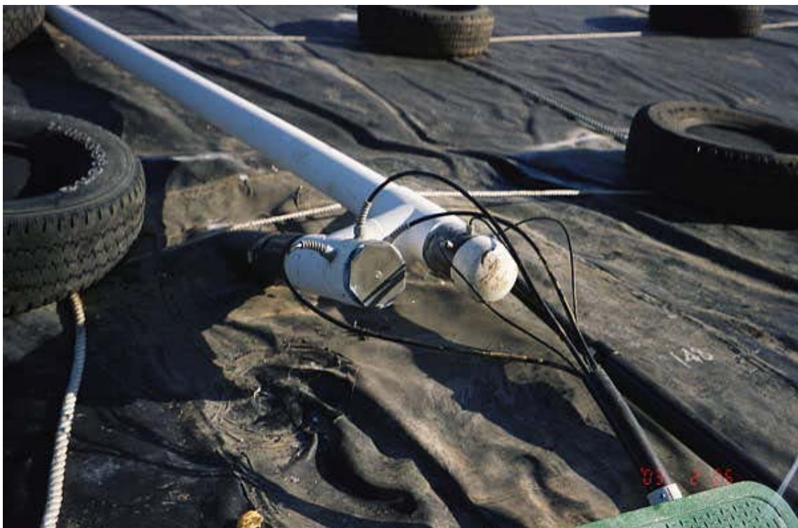
Image 44. Gas collection line on the northeast 3.5-acre area with fittings to allow sensor lines to exit the piping without leaks.
