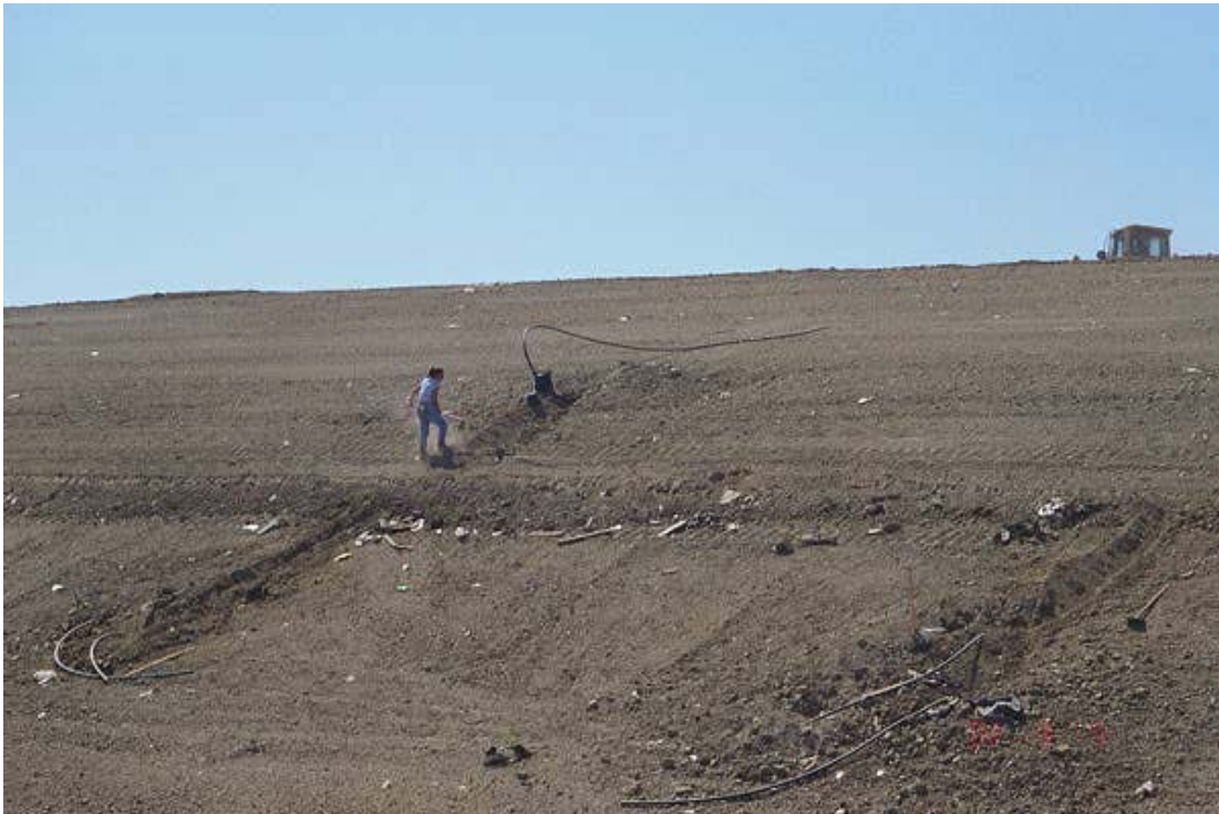
Image 6. Sensor wires were extended to the instrumentation shed and buried in the final cover soil layer. The entire module was then graded in preparation for geomembrane placement.
