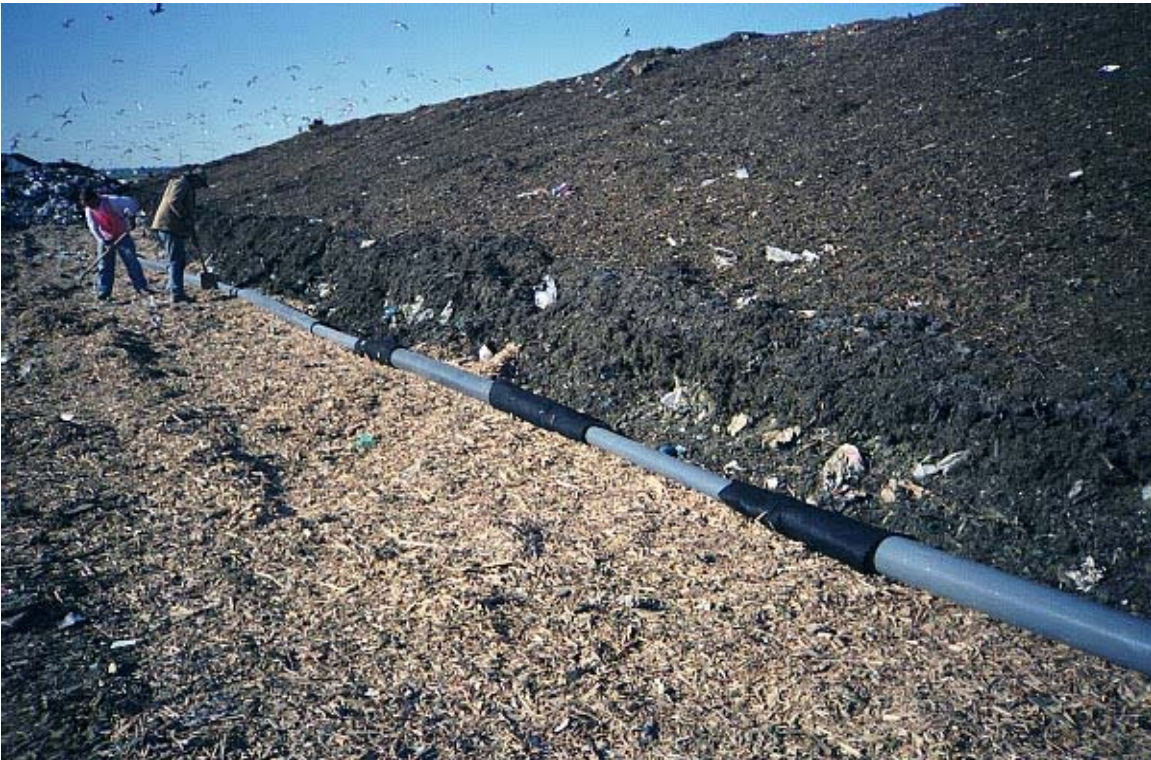
Image 21. Installation of the horizontal LFG collection line, with alternating 4 and 6-inch diameter PVC pipes. Filter fabric is wrapped over each joint.
