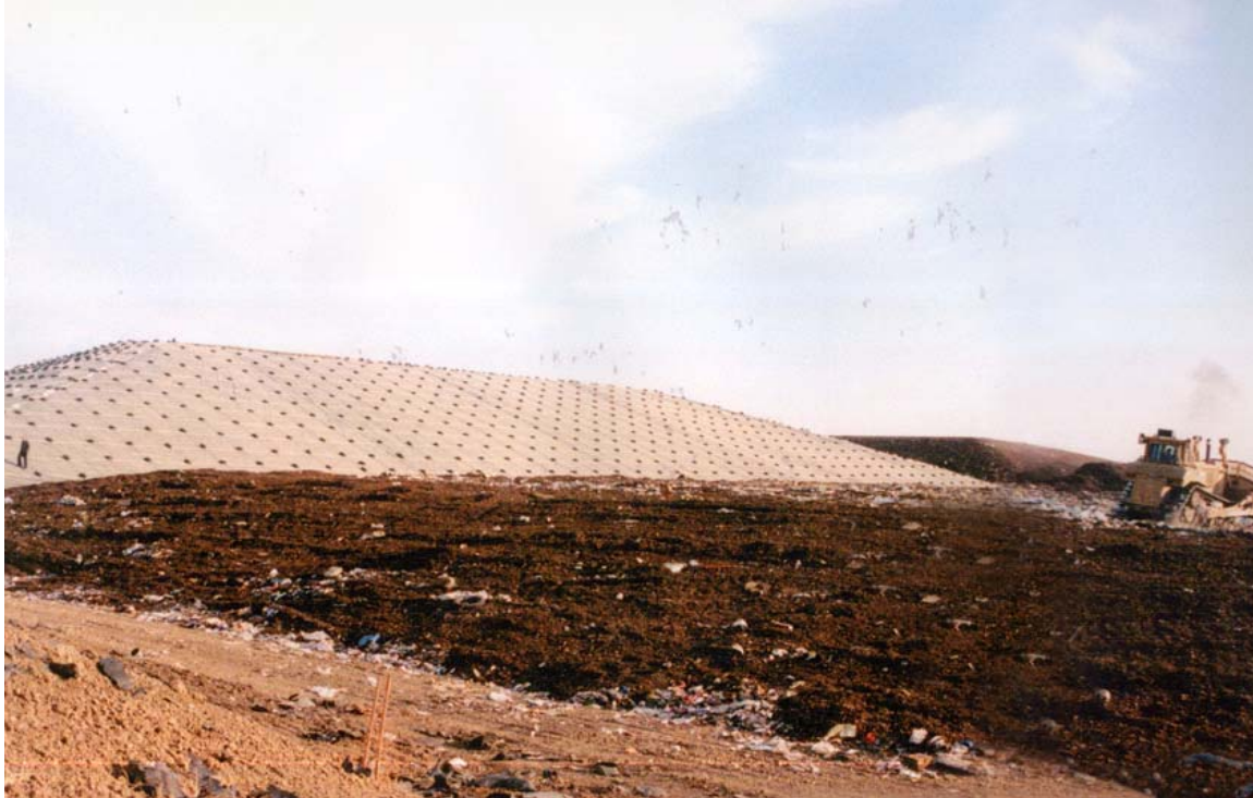
Figure ES-2. Northeast cell, shortly after geomembrane coverage, is in the foreground. The northeast cell footprint is approximately 300 ft by 500 ft, and it contains 78,000 tons of methane-enhanced waste. The scale is also indicated by a person walking up the cell cover near the lower left corner of the cell.
