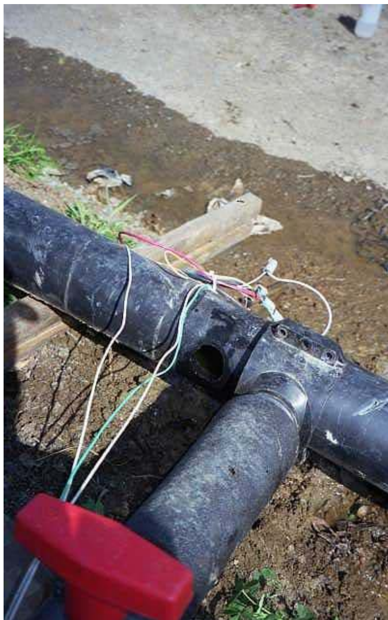
Image 39. Leak at saddle fitting between injection lateral and mainline. Saddle was removed and reinstalled with new gasket to repair leak
