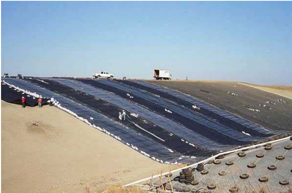
Image 31. Liner being deployed on the east side of the west 6-acre cell.
