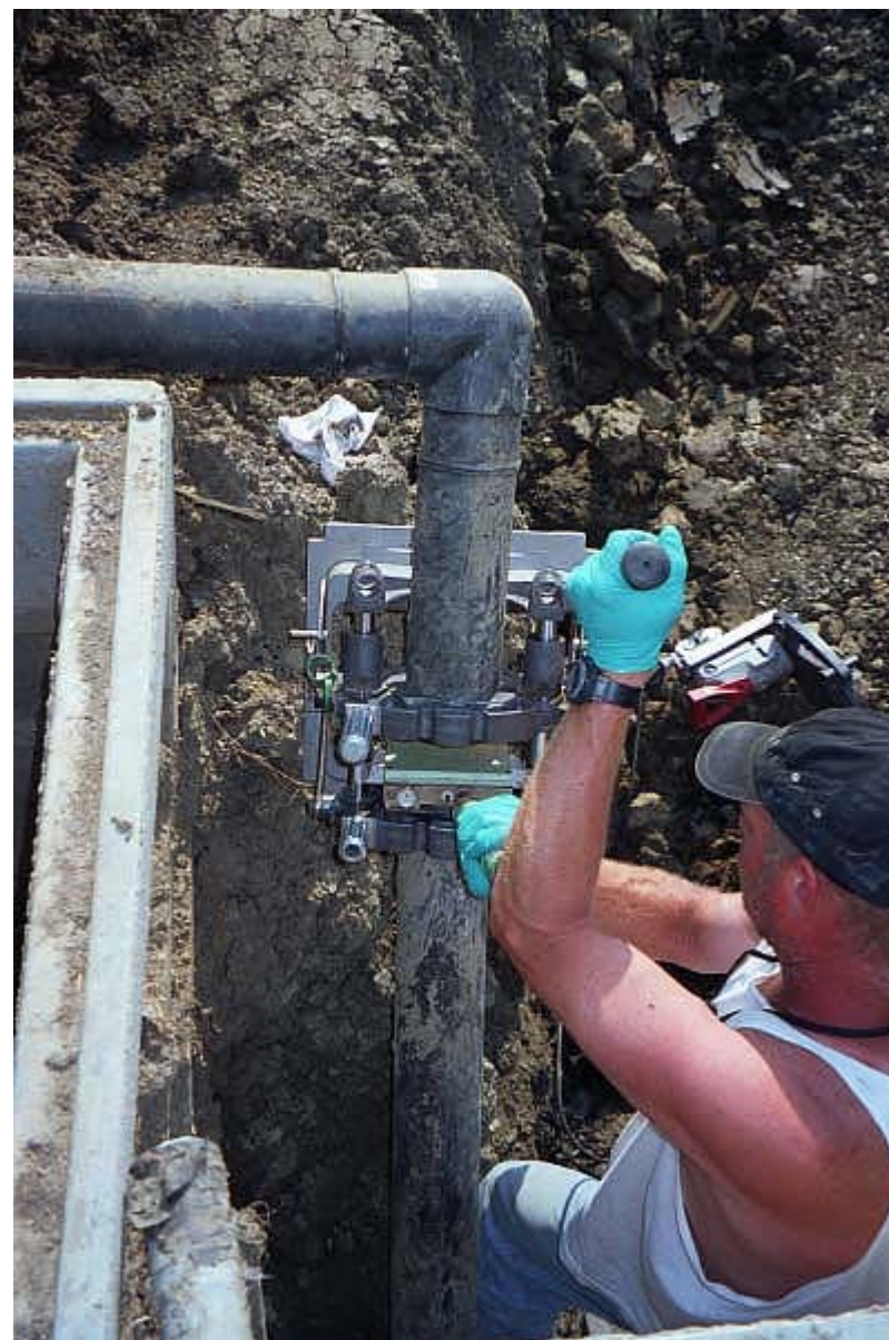
Image 40. Repair of leachate injection mainline. Pipe was cut at defective joint and re-welded by the butt fusion process
