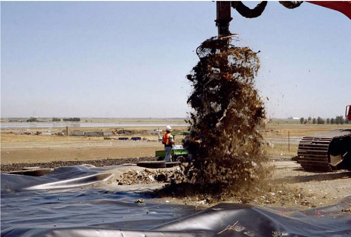
Image 37. Excavated waste was placed on liner material located adjacent to the boreholes where samples were then collected.
