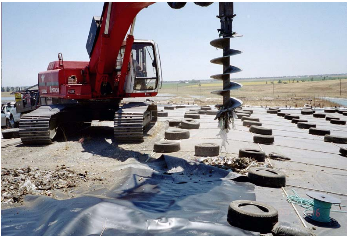
Image 36. An excavator-mounted drill rig was used for the sampling event to drill boreholes 25 to 40 feet deep.
