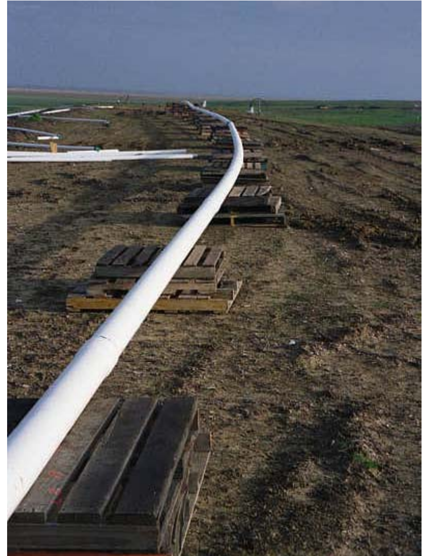
Image 24. Recycled pallets were used on the gas collection header line to establish the necessary slope to allow condensate to drain.
