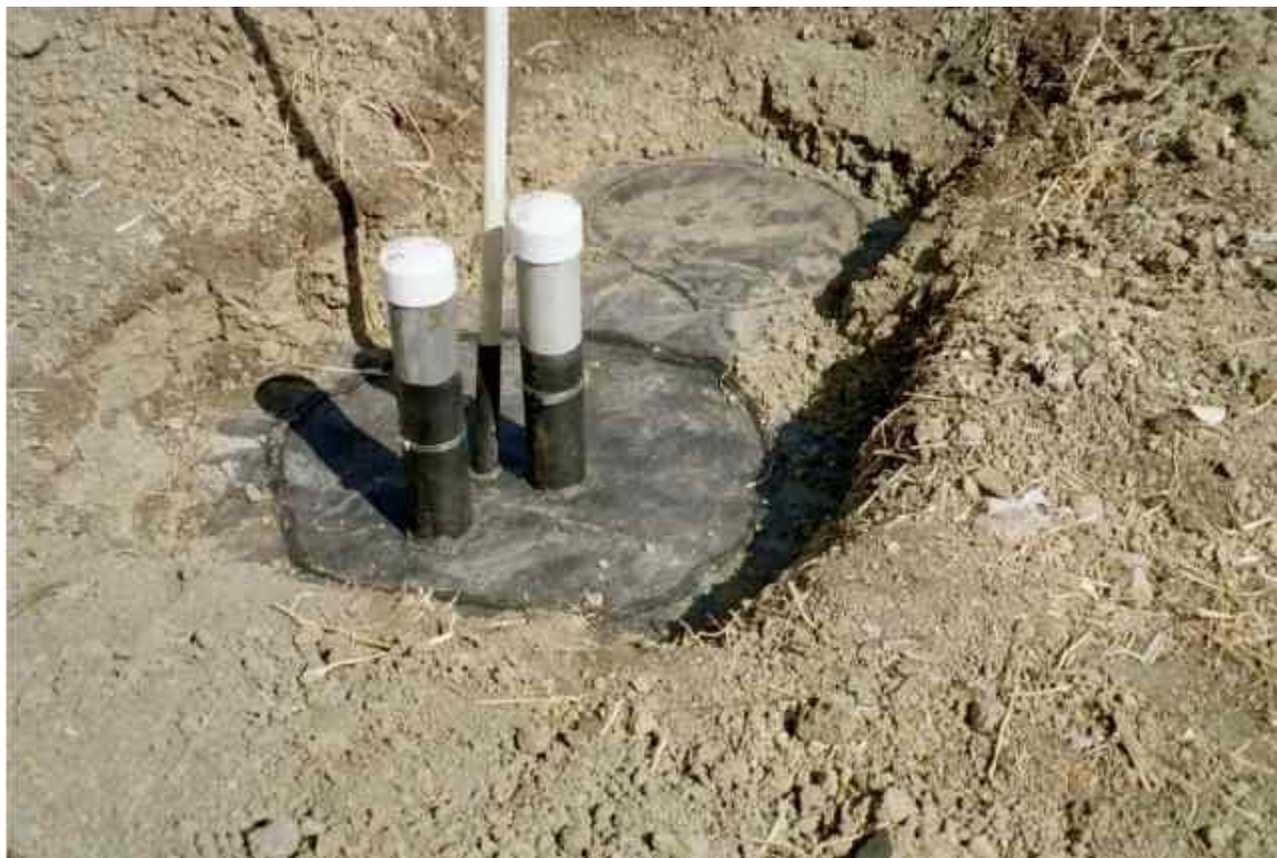
Image 46. Vertical gas collection lines installed on west 6-acre cell.
