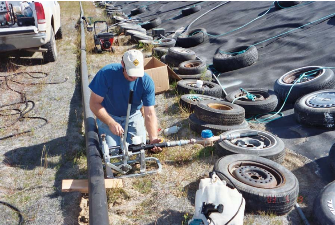
Image 20. Injection laterals were fusion welded to the 4-inch diameter HDPE injection header to minimize the possibility of leachate leaks.
