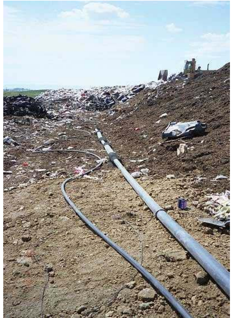
Image 18. Soil bedding was used where the injection and gas collection lines exited the waste. The lines were then covered with soil to encapsulate them and to minimize the possibility of leachate seeping out of the cell
